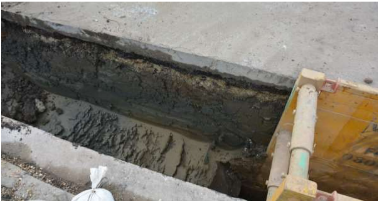
Fig.5: Open-cut trenching outside No.26 Brindwood Road facing SSE, showing natural clay at base
