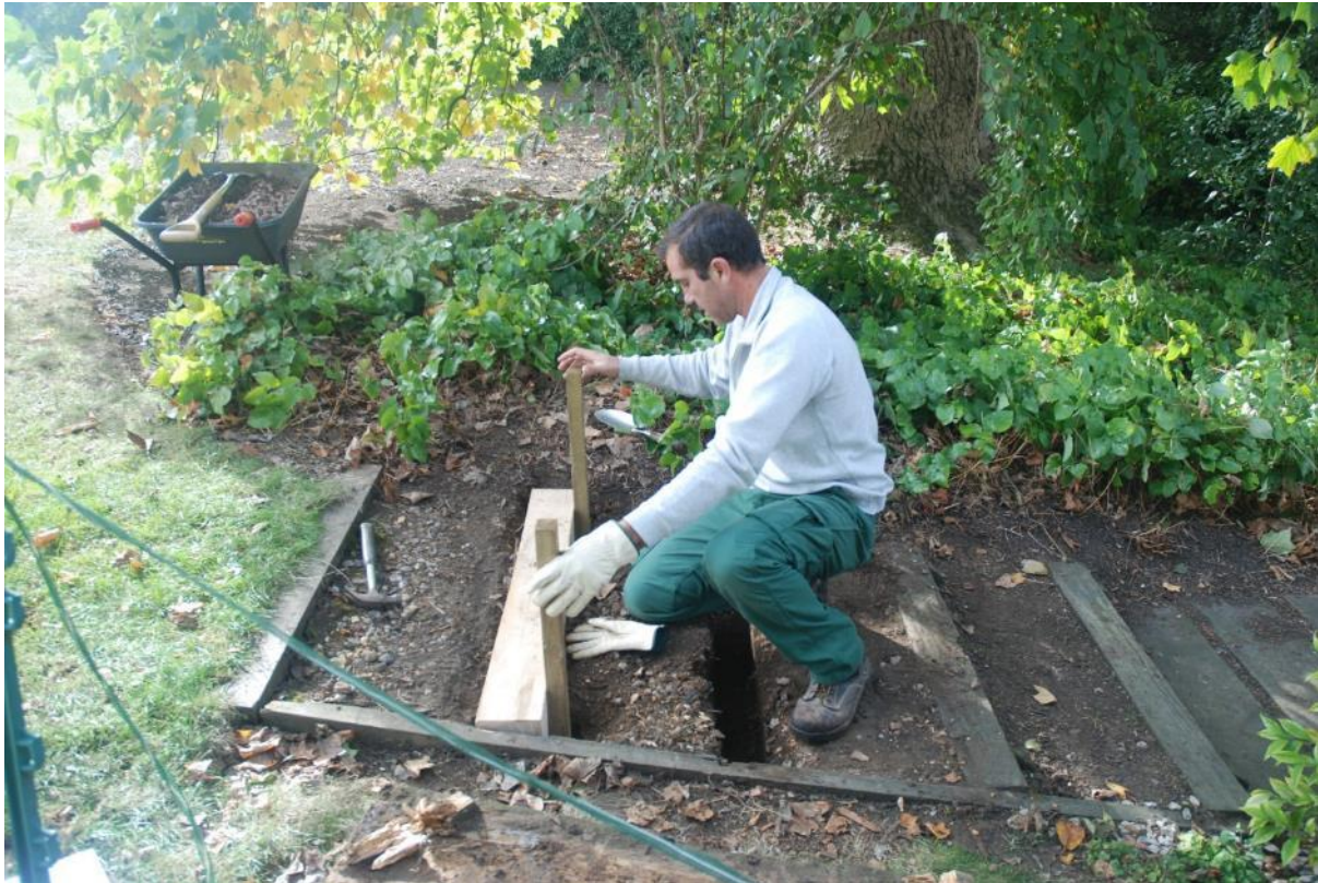
Figure 7: Working shot showing the installation of the new steps in the trench created by the removal of the old. Facing S. No scale.
