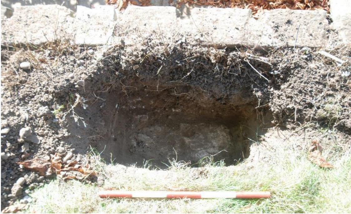
Figure 12: Pit 5, east of Pit 3 above. Concrete foundations for the wall seen at the top of the frame can be seen at the trench base. Facing S. Scale 0.5m.
