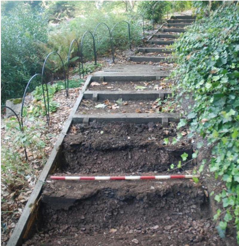
Figure 4: Post-removal of boards from the 10th and 11th steps (from the bottom of the flight). Facing NE. Scale 1m.
