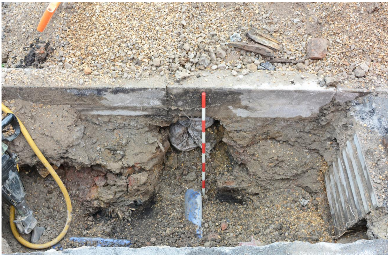
Fig.3: Detail of the south-east section. The dark areas at the base represent localised organic silt deposits, cut & truncated by modern activity
