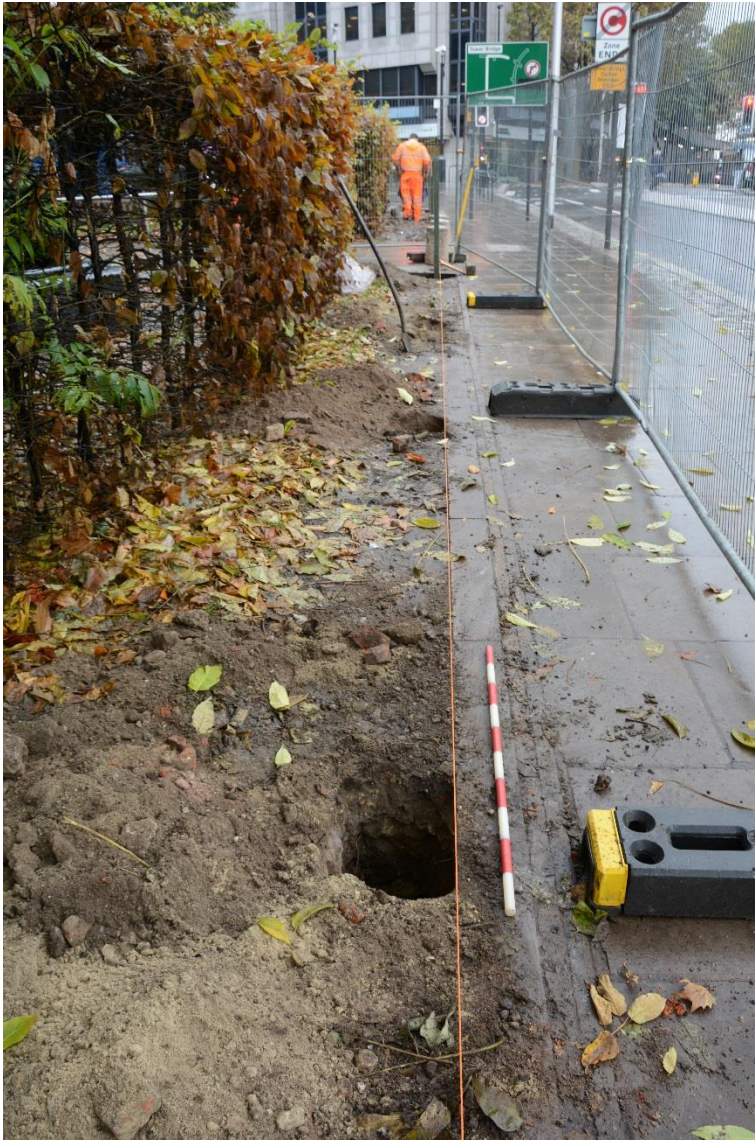
Figure 8: B: The above trenches, as seen from the western end, facing towards Minorities. The new railings were installed starting from the east end, moving towards Tower Hill station. Facing NE. Scale 1m.
