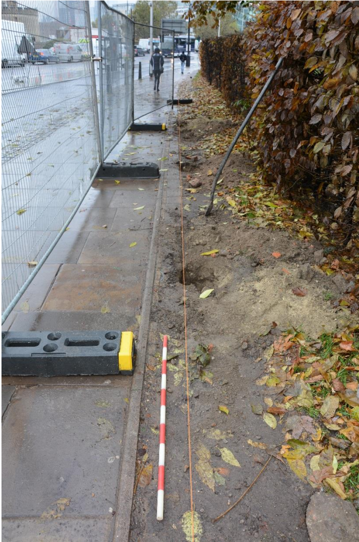
Figure 7: A: Four open pits to the west of the southern entrance. Facing SW. Scale 1m.
