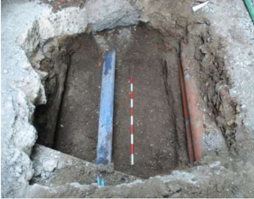
Figure 5: Tree pit one showing water main [5]/(6) through centre and modern services [3]/(4) on right side. Facing NE. Scale 1.0m
