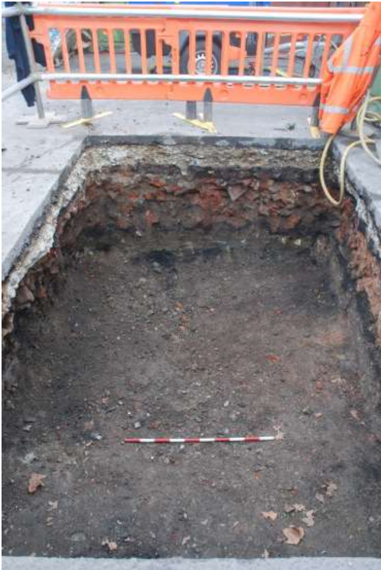
Figure 7: Completed trench, showing backfill below modern car park surface. Facing NE. Scale 1m.
