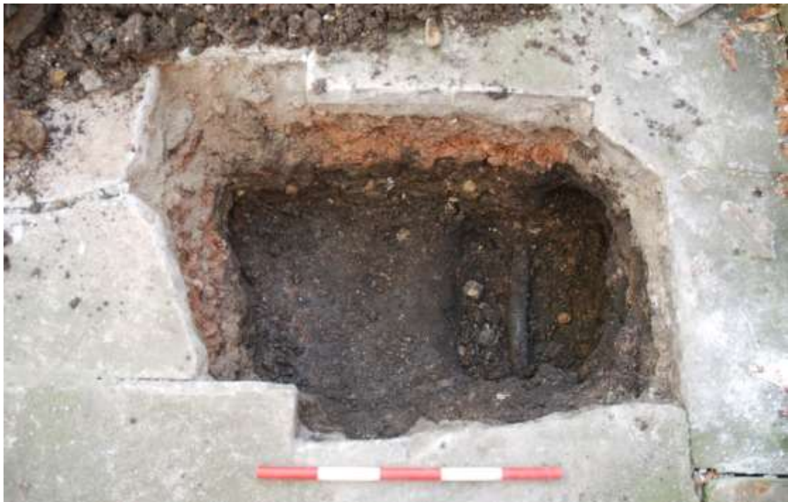
Figure 6: Pit 6, showing backfill below MOT Type 1 and existing paving. Facing E, scale 0.5m.
