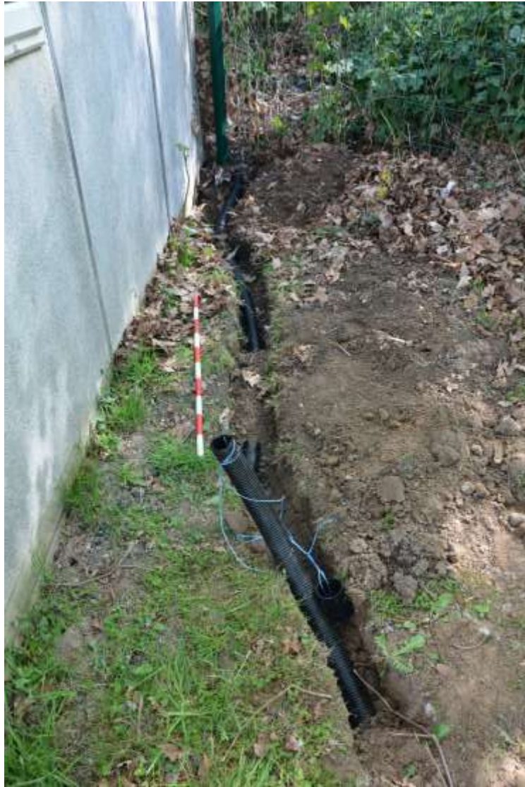
Figure 16: Portion of cable trench near SE corner of hutted classroom facing E, 1m scale
