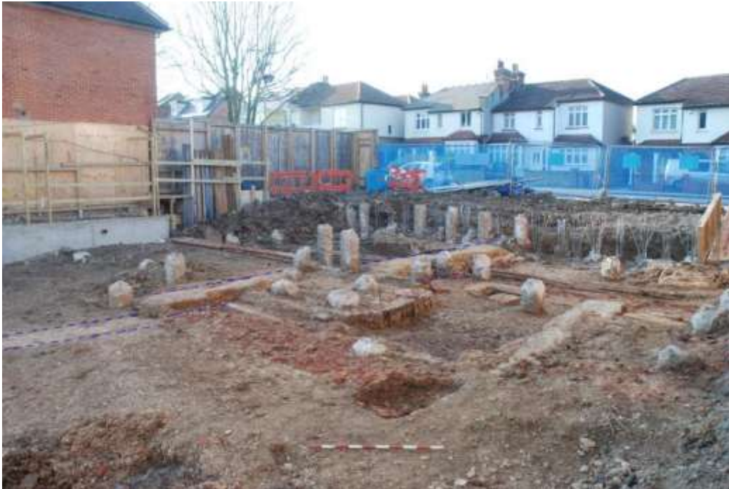
Figure 37: Wall [53] (marked in blue) seen running N-S through the centre of site. Facing NW. Scale 1m.
