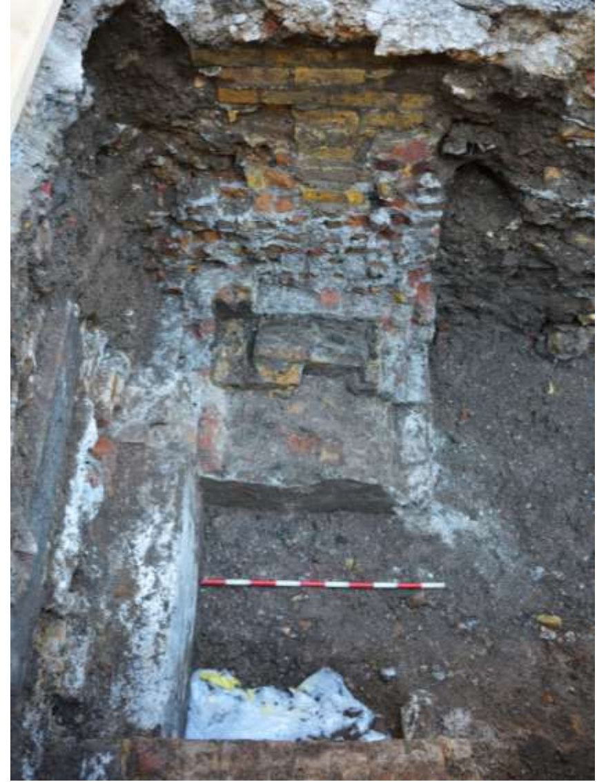
Figure 5: The sewer [50], northern end of the drop shaft. Looking E. Scale 1m
