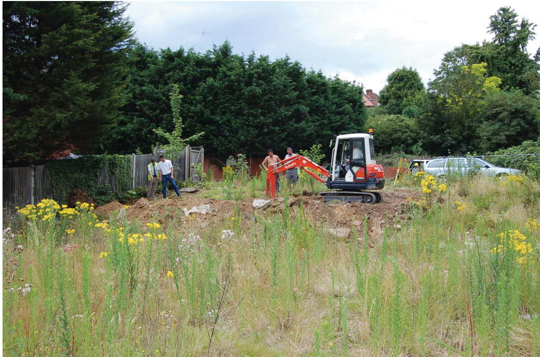
Fig 7 A view of the groundworks, looking back northwards from the Brighton Road frontage. The artificial mounding of the deposits on site can be seen. The machine stands in approximately the area where the terracing for the old house had its northernmost limit.
