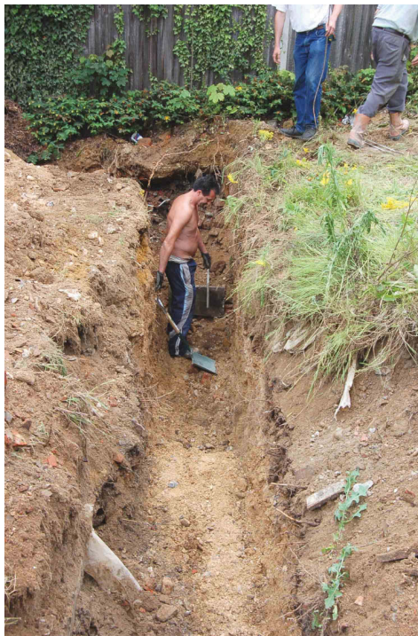
Fig 6 General view of the groundworks excavations looking southwest along the long axis of the groundworks trench. Modern made ground deposits were exposed in this area to a depth of 1.8m below current ground surface (where the figure is standing in the trench).
