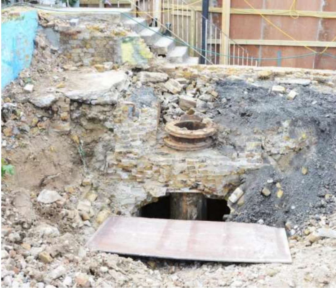
Figure 26: View of the chamber with capping removed. The standing walls of the old pump-house are visible to the left and rear of the chamber (partially demolished during works). Looking S. No scale.
