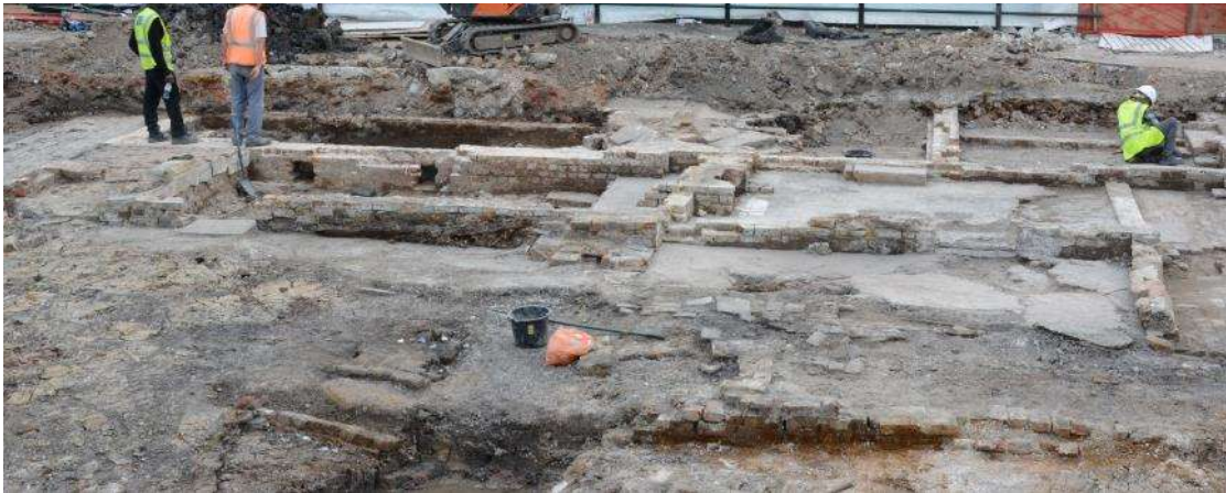
Figure 59: Working shot of back yard with concrete surface (45). Structure [47] visible unexcavated in the foreground. Looking SE. No scale.
