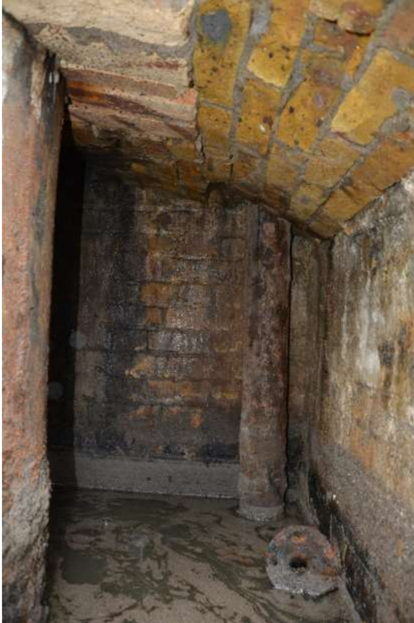
Figure 28: Interior southwest corner of chamber showing secondary downpipe and pump head. Arched ceiling and standing water visible. Facing S. No scale.
