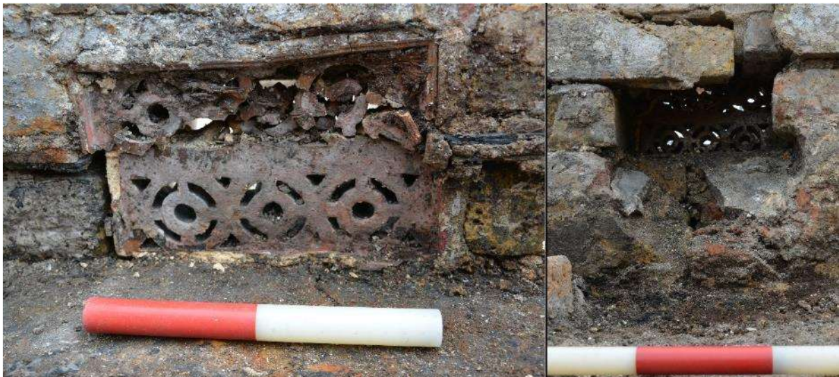
Figure 51: Ceramic grilles set in to [30]. Left: facing SE, scale 0.2m; Right: facing NW, scale 0.1m
