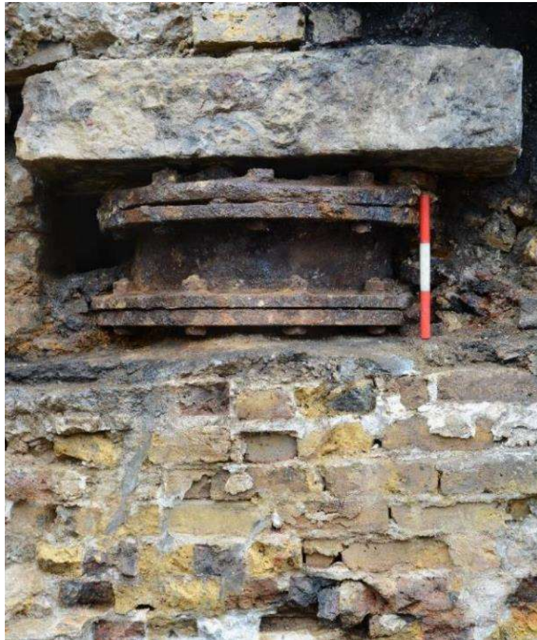
Figure 27: Detail of flanged separator section of pipe with NW twist. Concrete capping above and remainder of pipe extending into chamber below. Facing S. Scale 0.3m
