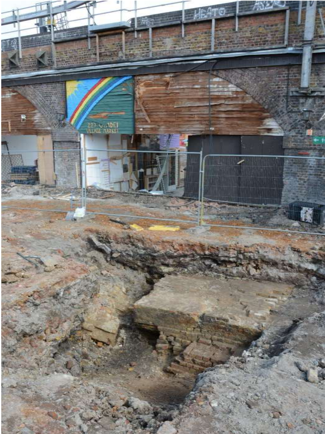
Figure 35: Working shot of the railway associated structures [1], [2] & [4], showing proximity to present-day viaduct. Looking NW.
