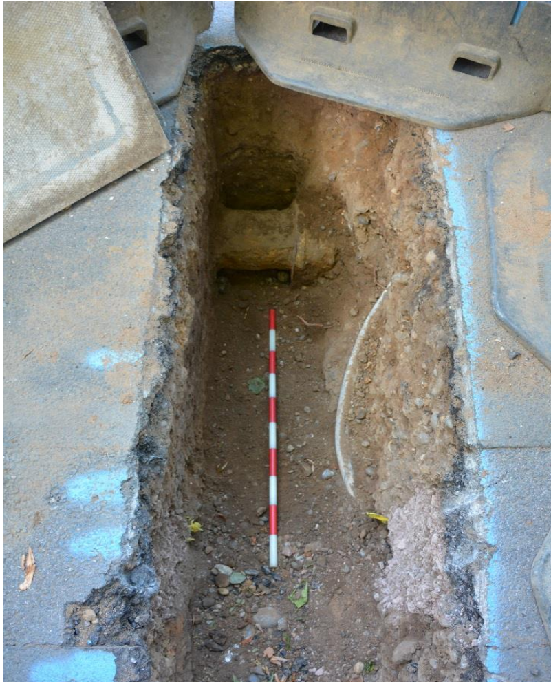
Figure 8: Western part of Trench 2. The continuation of the main can be seen towards the top of the frame, and service cut [7] towards the bottom. Facing W. Scale 1m.
