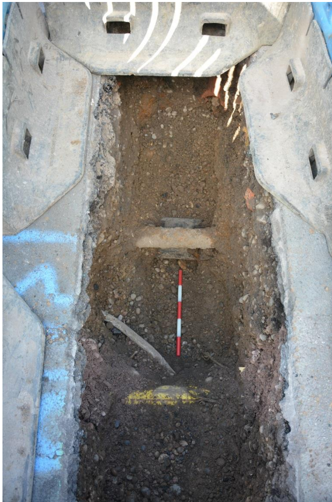
Figure 12: Trench 4, showing N-S services below modern made ground. The remains of a ceramic drain can be seen towards the top right of the trench. Facing W. Scale 0.5m.
