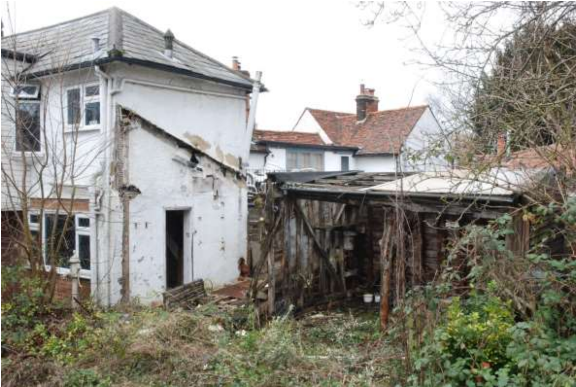
Fig.60: Exterior of eastern elevation, note the 'scar' of the sloping roof of room G5
