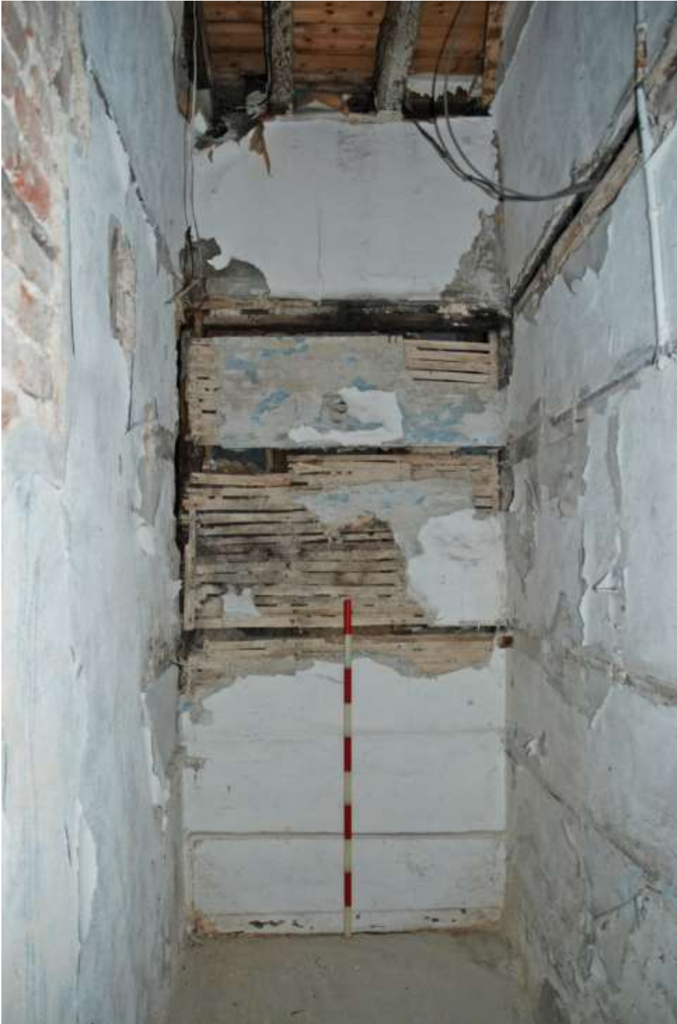
Fig.47: Cupboard room G3, facing W, 1m scale. Note the lath and plaster construction of the west and north walls and timber / brickwork of southern wall
