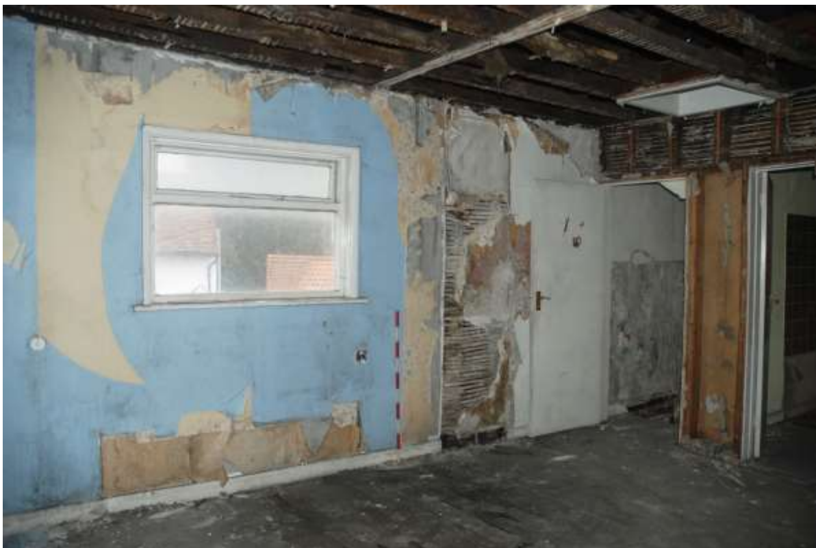
Fig.72: Room F1 eastern extent indicated by the lighter timber in the ceiling and end of blue wallpaper, facing NE, 1m scale
