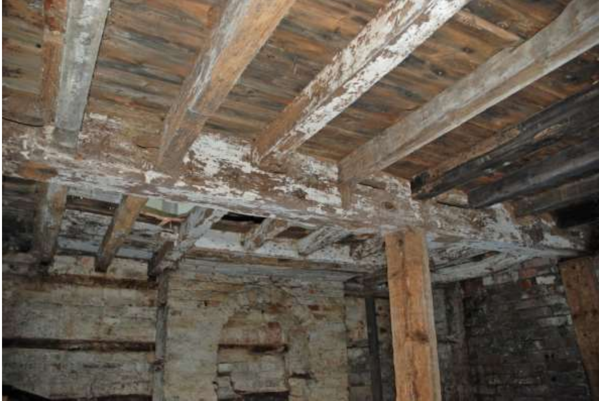
Fig.24: Detail of the cellar ceiling. Facing towards the SE corner. Note the earlier beam with empty mortices compared to the extant modern, machine cut joists and boards
