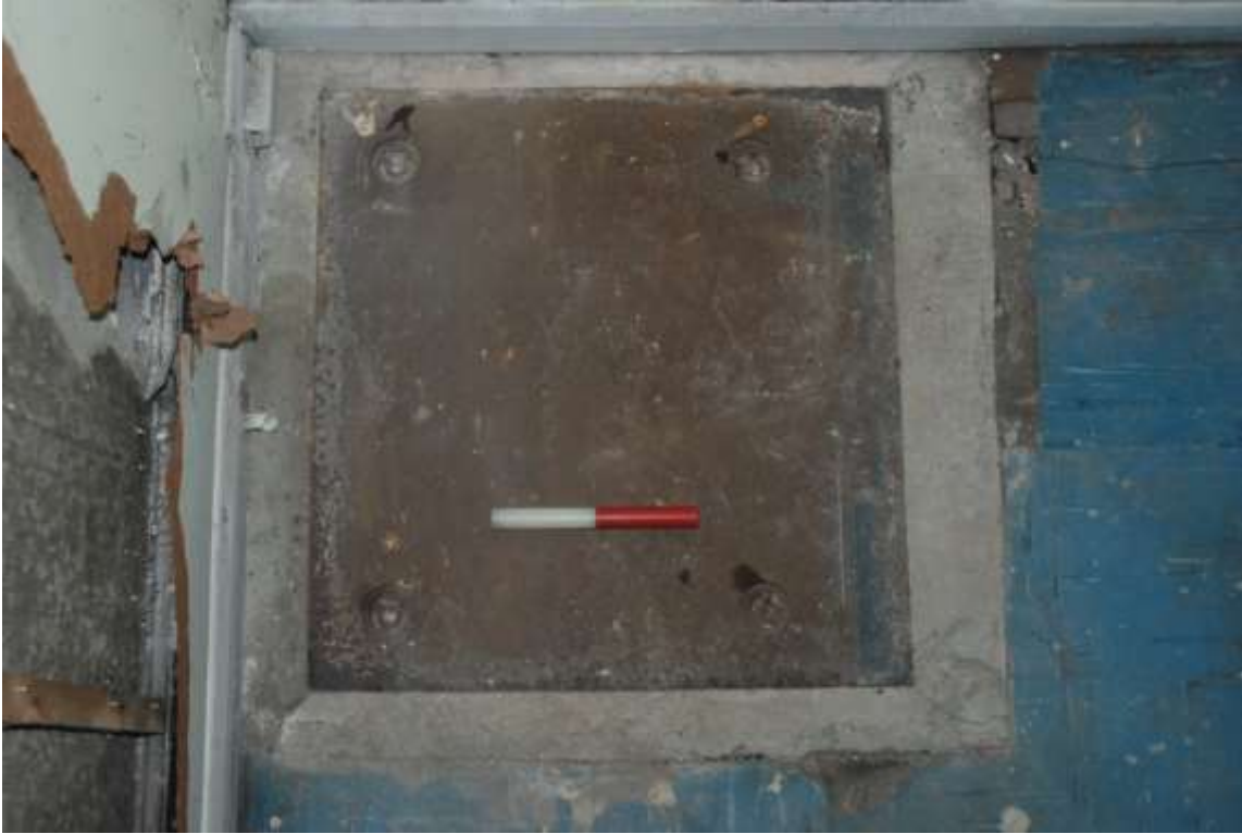
Fig.37: Floorplate for the boiler in the southwest corner of room G1, facing W, 0.20m scale
