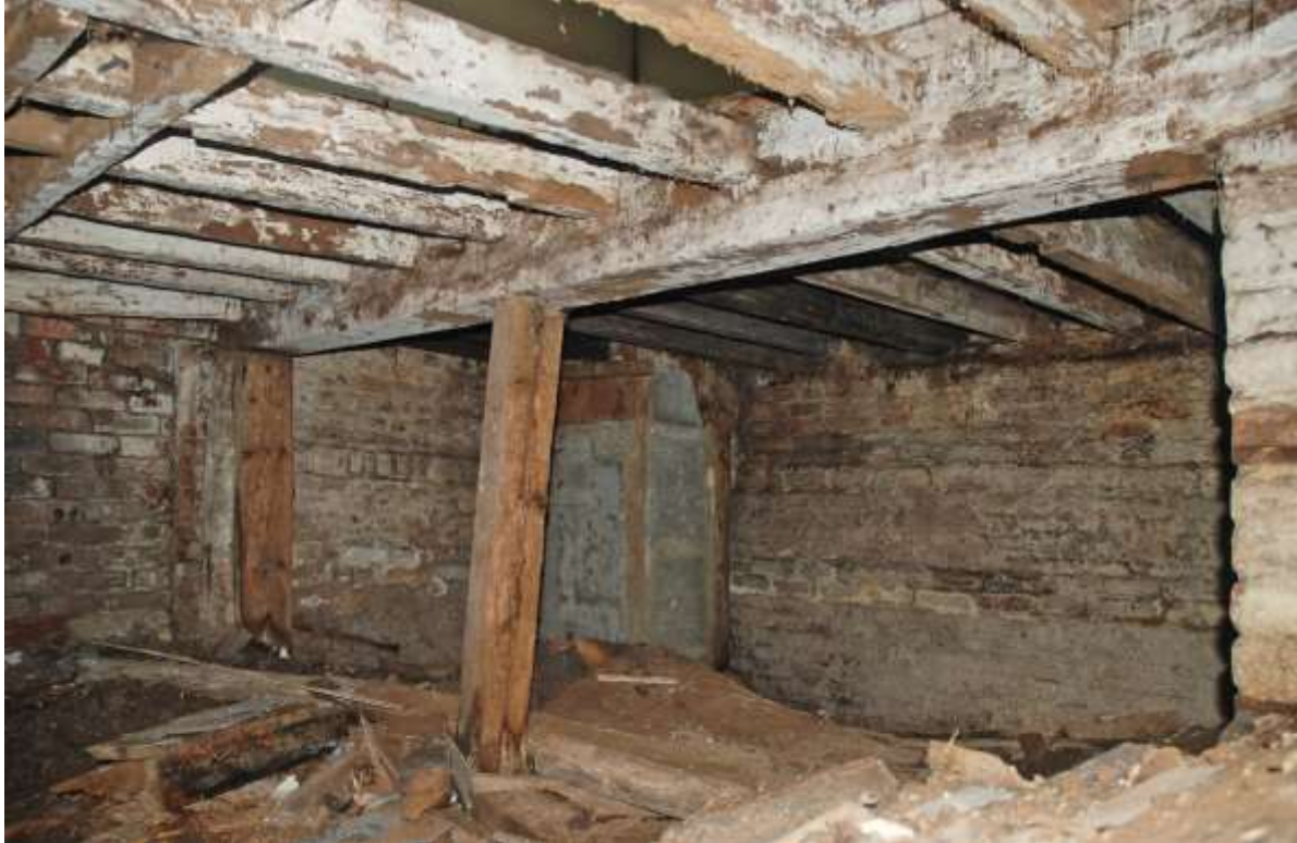
Fig.23: Southwest corner of the cellar showing concrete block base for boiler. Facing SW
