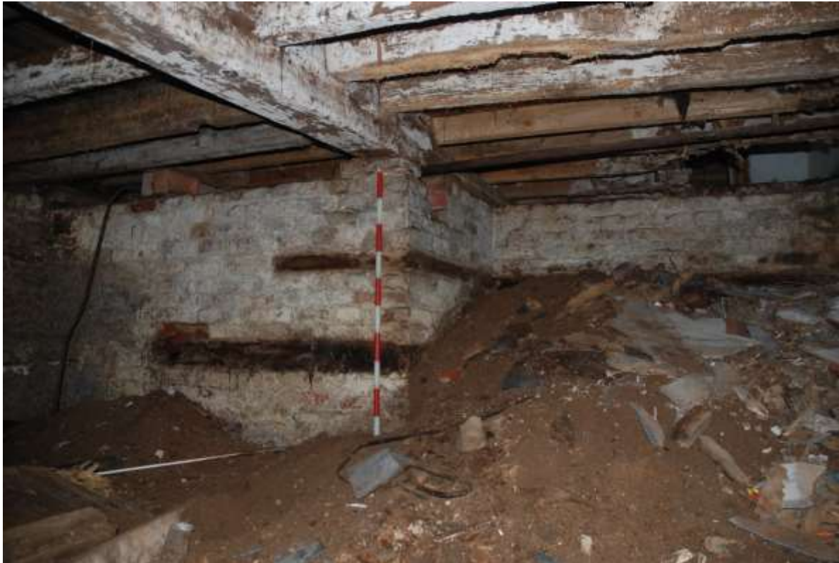
Fig.18: North wall of the cellar with projection and bond timbers, facing NNW, 1m scale
