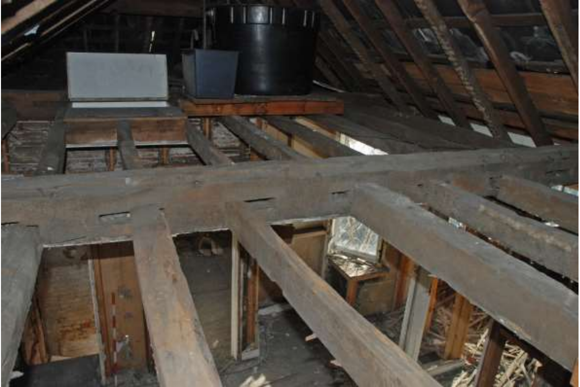
Fig.105: Roof space over room F1, facing ESE, towards eastern end and water butt over room F2, (bathroom). Note reused central beam with empty mortices and cut outs
