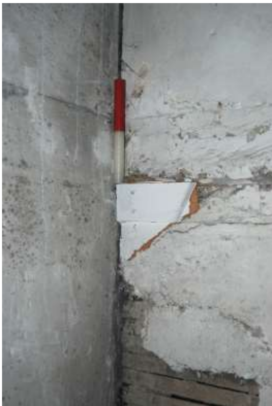
Fig.44: Northeast corner of room G2, facing NE, 0.20m scale. Note gap between abutting east wall and plasterwork of north wall continuing beyond into room G4
