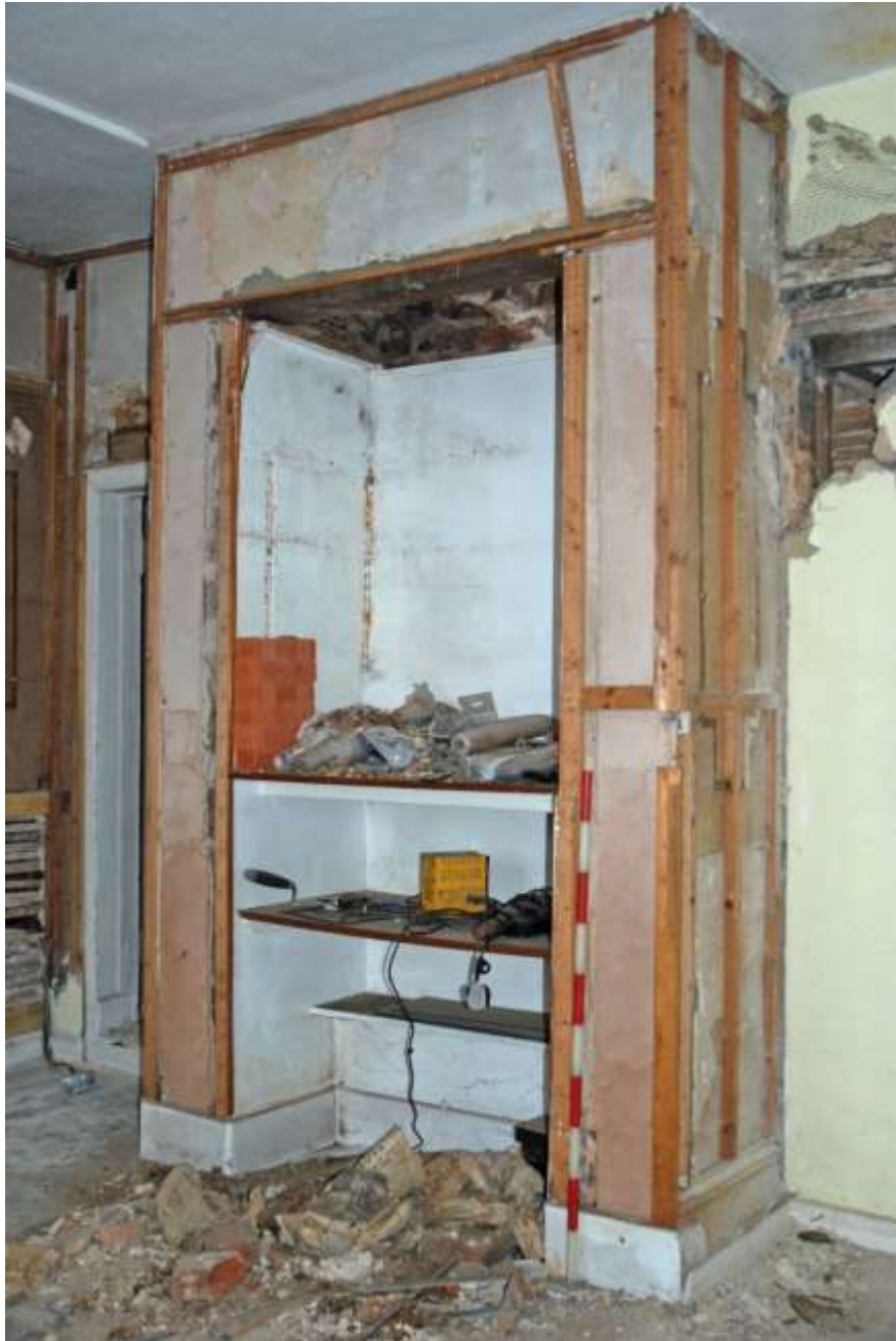
Fig.32: Former fireplace in northeastern corner of room G1, facing NE, 1m scale
