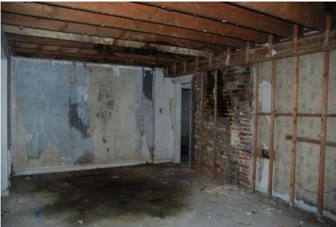
Fig.62: Room G6 facing SW showing door to room G1 in the corner of the room and sooting of former fireplace. The southern wall is breeze block behind the plasterwork
