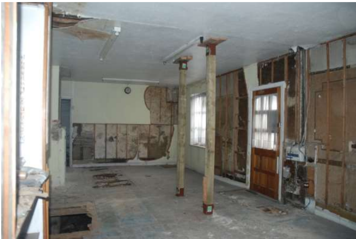
Fig.29: Room G1, facing SW, showing former decorative schemes on the south and west walls. 'Scars' of former hallway walls along the ceiling
