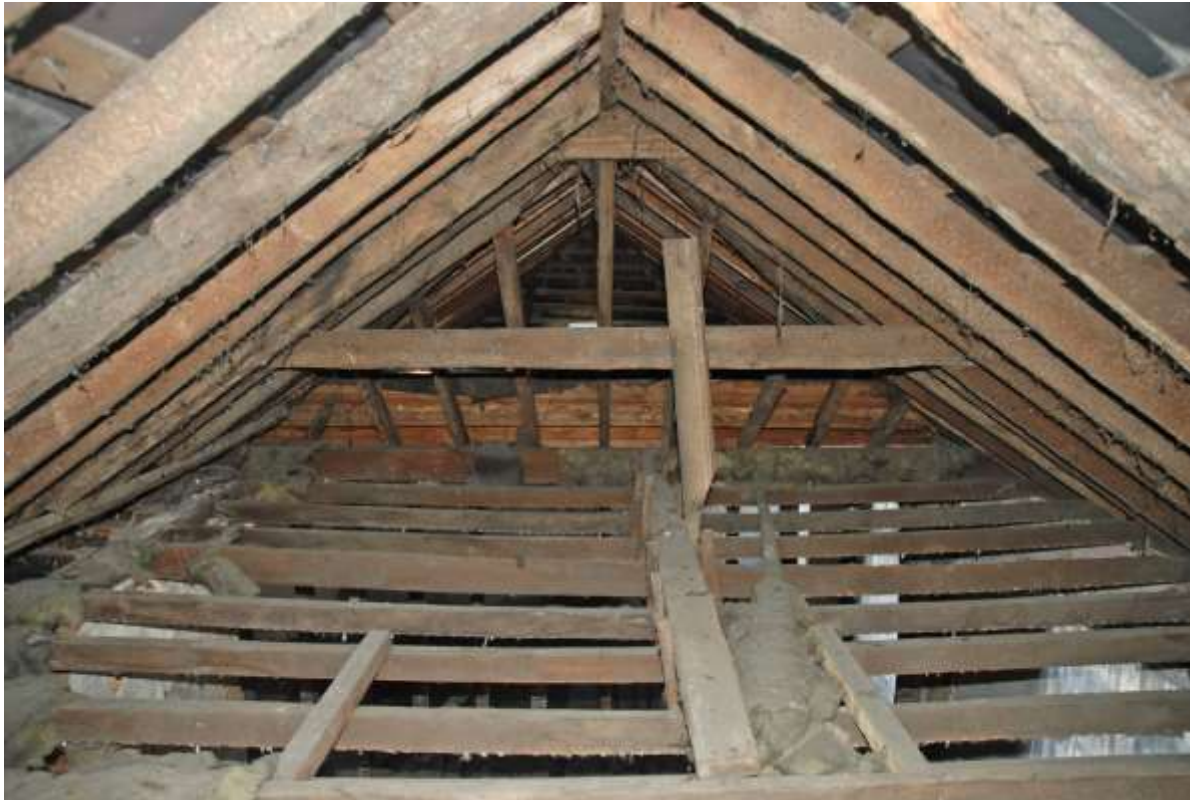
Fig.100: Roof space over room F4, facing S towards original hipped end of roof, and to southern extension beyond
