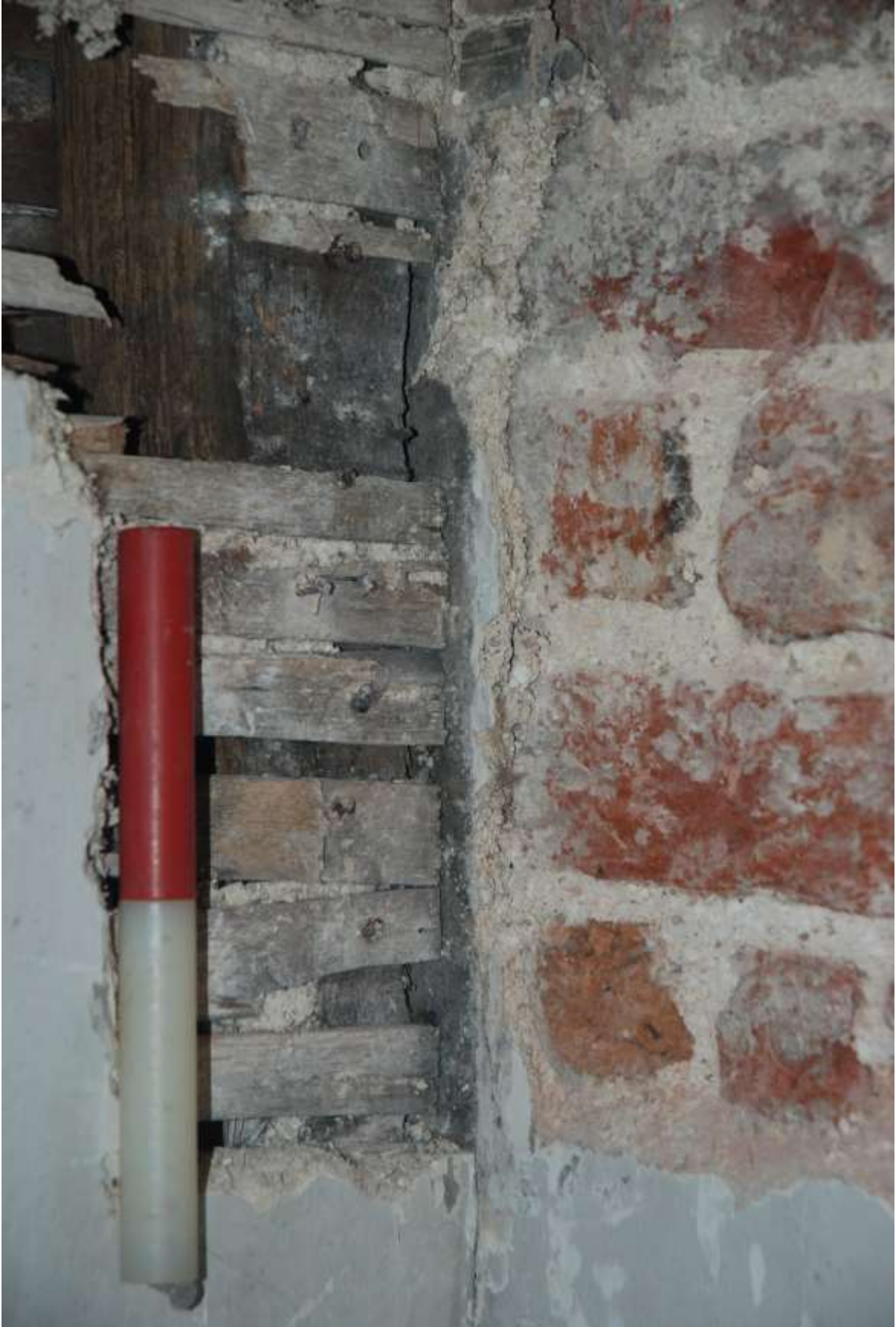
Fig.45: Detail of lath and plaster abutting rear of chimney stack in the SW corner of room G2
