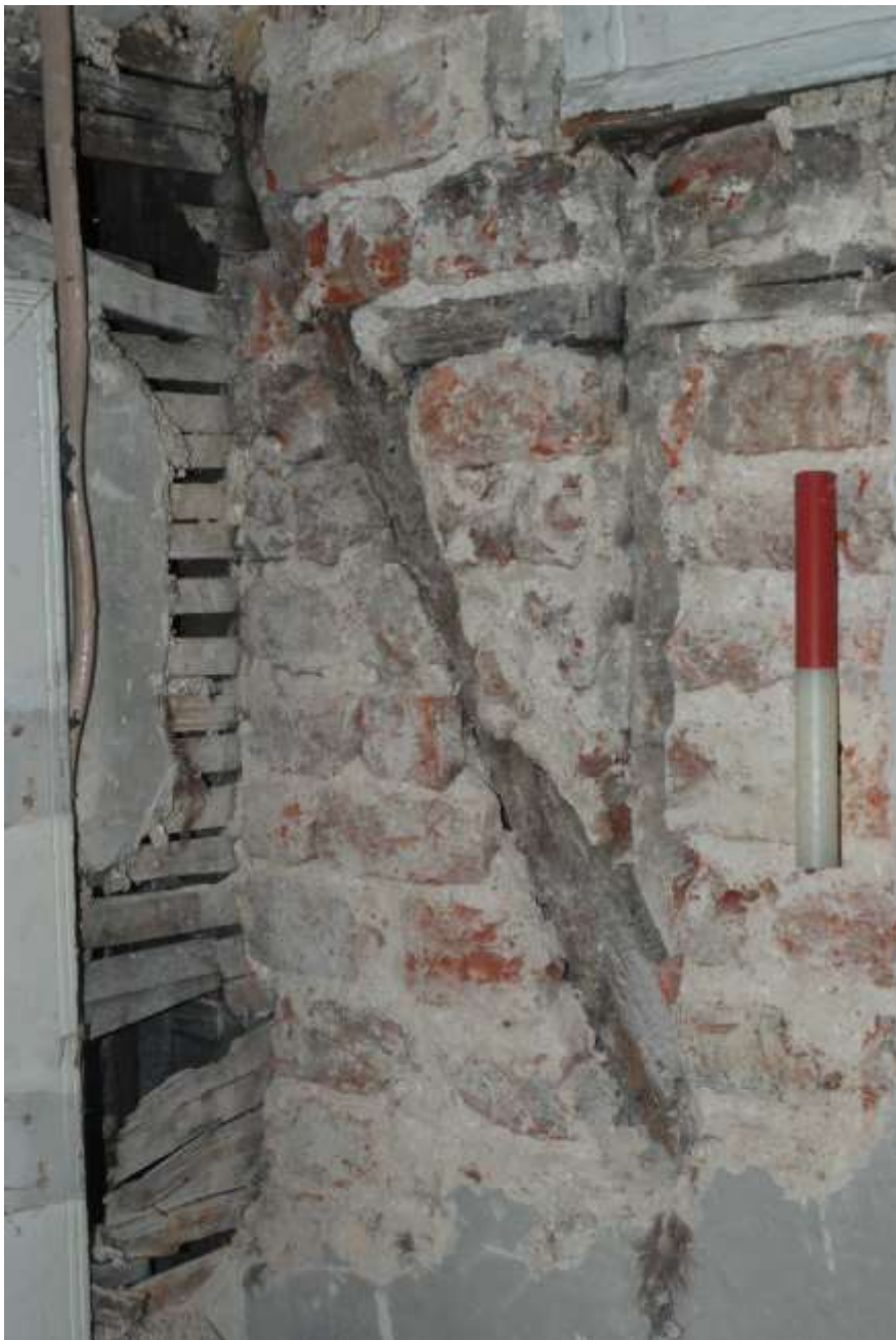
Fig.42: Northern wall brickwork bonded to and overlying lath and plaster work of western wall, facing NW, 0.20m scale
