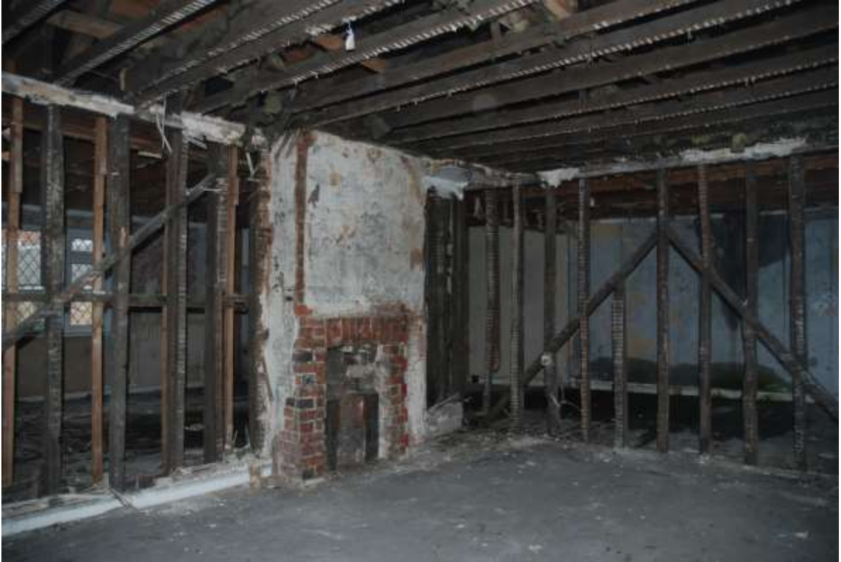
Fig.84: Room F4, facing SE into rooms F5 and F6 beyond timber framework, 1m scale
