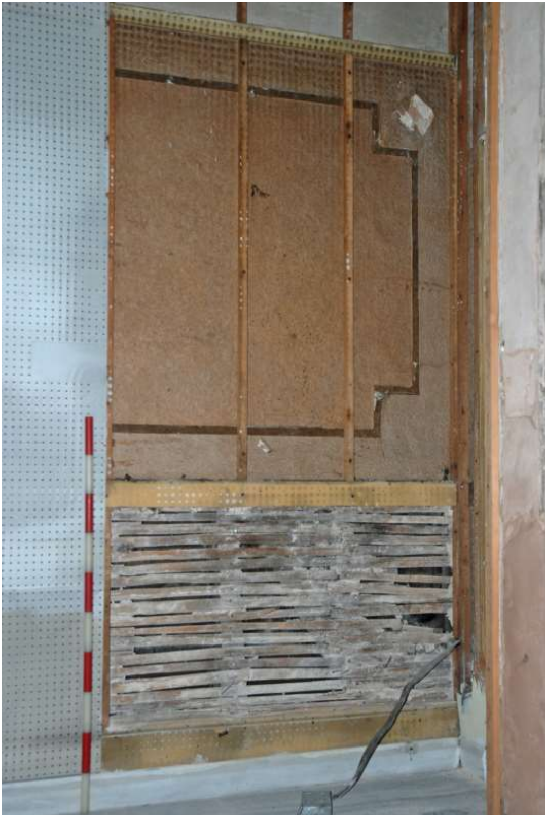
Fig.38: Northeast corner of room G1, facing N, 1m scale. Detail of former decorative schemes and lath and plasterwork construction visible
