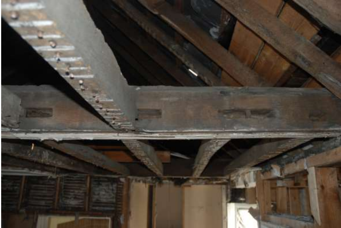
Fig.75: Detail of the eastern face of ceiling beam in room F1, towards southern wall and valley of roof showing the empty cut outs / mortices. The one on the right retains a peg / dowel
