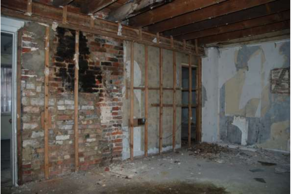
Fig.65: West wall of room G6, facing NW showing the sooting of former fireplace
