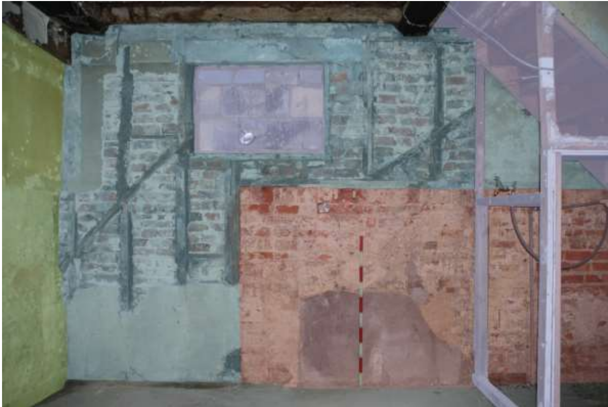
Fig.53: Marked up photo of the north wall, facing N, 1m scale. Green earlier phase of building, Red first phase of brickwork, blue secondary phase with the infilled timber framing. Purple represents modern intrusions, infilling of window and stairs
