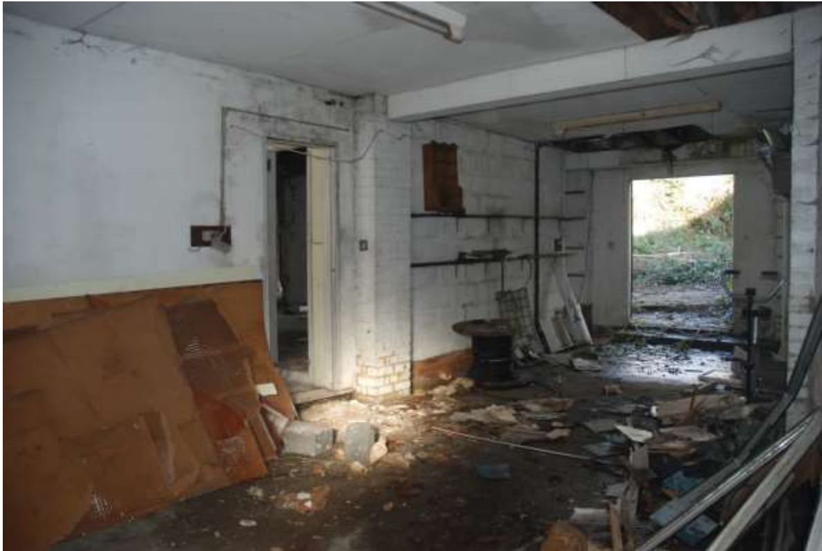
Fig.67: Garage space facing NE, access to GI in centre left of frame and door to garden in background. Note the breeze-block construction in NE corner and the northwest original external wall
