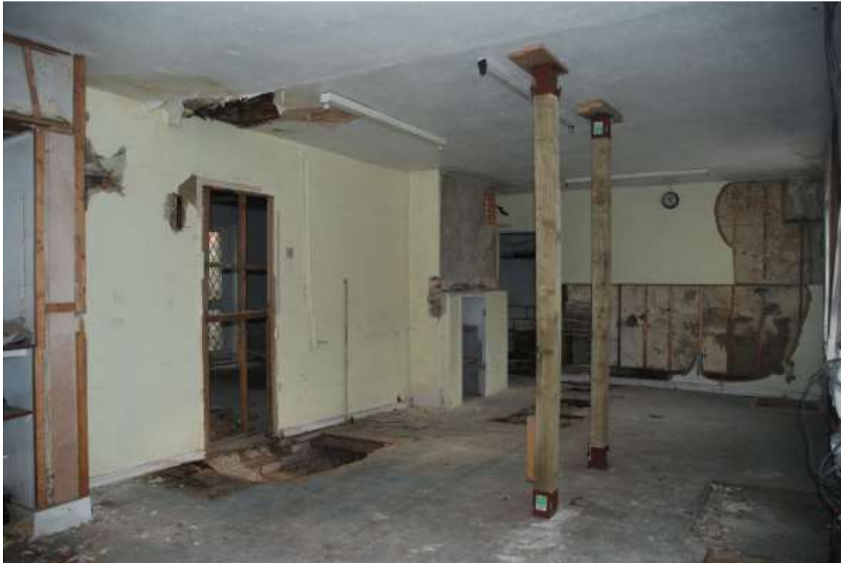
Fig.28: Room G1, facing SE, showing north fireplace / cupboard in left of frame. Southern fireplace / cupboard in background. View down into cellar and into back room in centre
