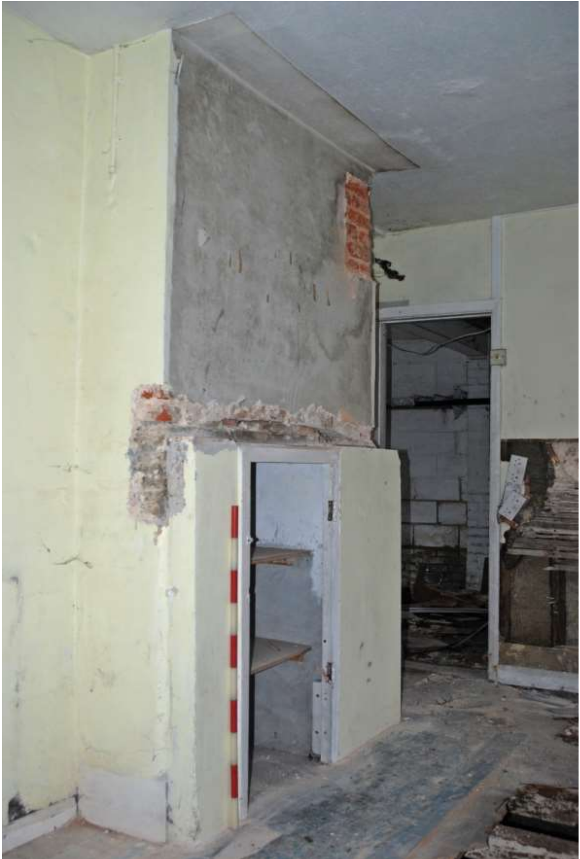
Fig.34: Former fireplace in the southeast corner of room G1, since converted into a cupboard and safe, facing SE, 1m scale. Note the exposed original brickwork in the upper portion.
