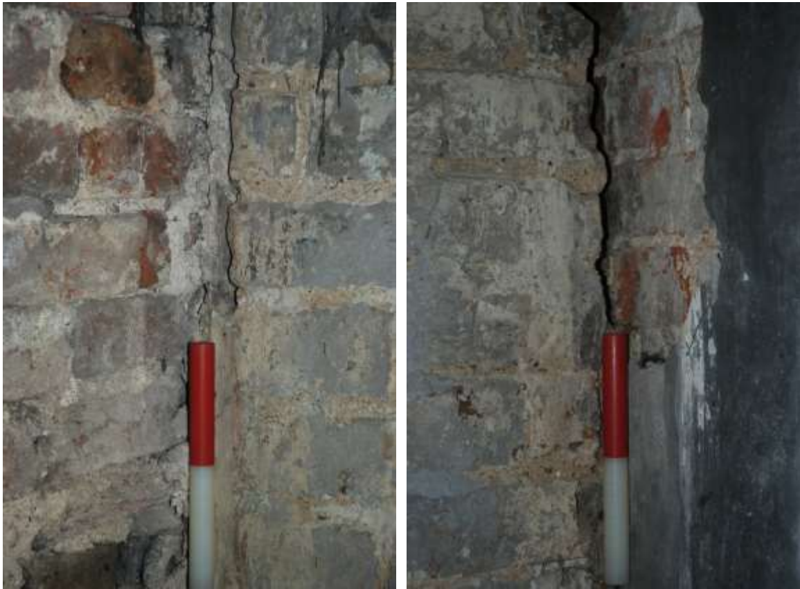
Fig.55: Detail of the NE, (left), and SE, (right), corner of Room G4 showing the lack of bonding between the eastern wall and its north and south counterparts, 0.20m scale
