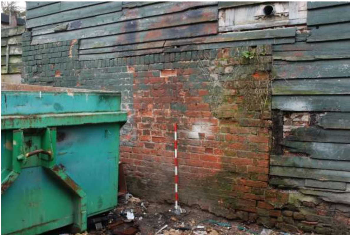
Fig.15: Northern elevation, eastern end, solid brickwork also visible in room G4, facing SE, 1m scale. The brickwork probably formed part of an original boundary wall, later utilised in the eastern extension / remodelling of the property
