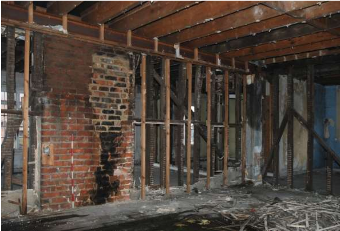
Fig.93: Room F5 facing NW, showing the sooting on the rear of the southern fireplace, and RSJ at ceiling height
