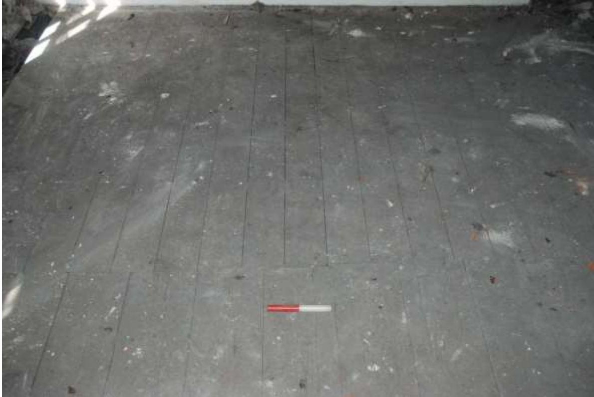
Fig.89: Detail of the change in floorboards over the area of the hypothetical original staircase, facing N, 0.20m scale
