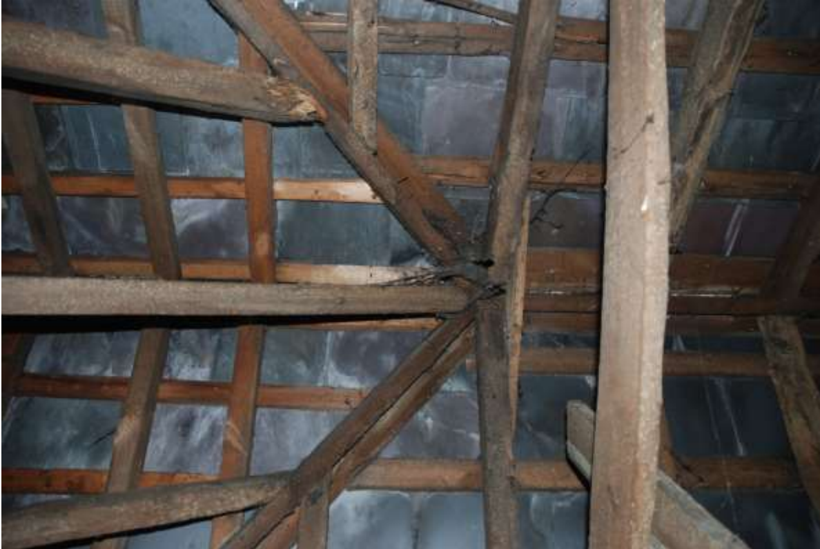
Fig.102: Roof space over room F4. Southern end looking directly up at original hipped end of roof, since remodelled to accommodate southern extension, (see fresher timbers on left of frame)
