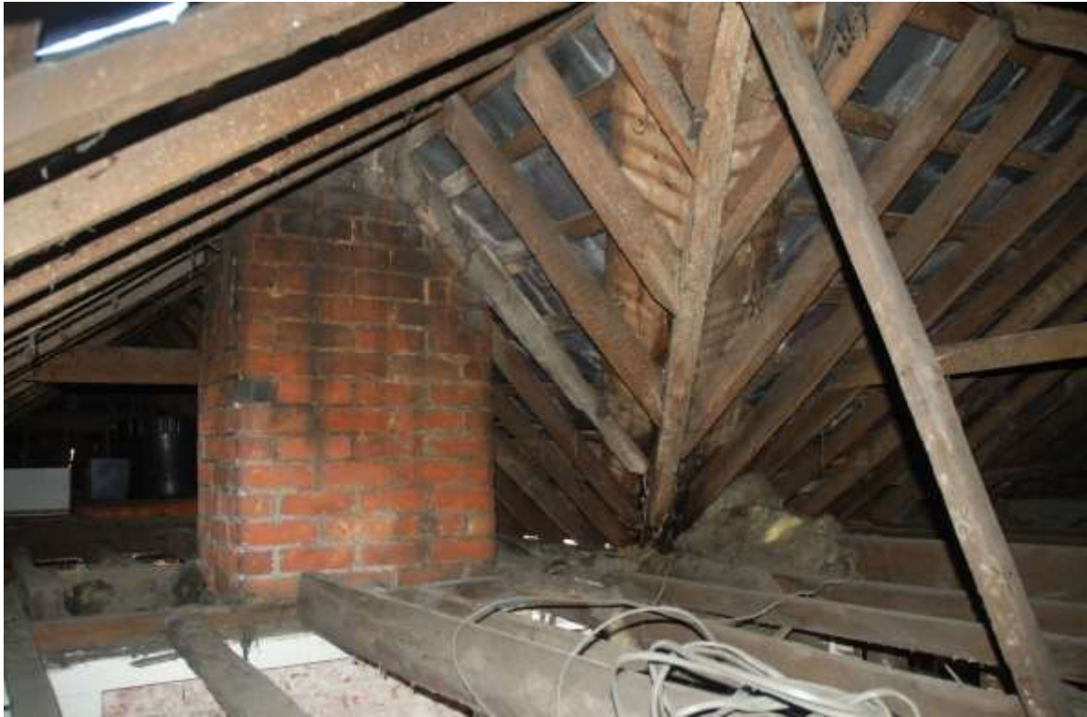
Fig.103: Roof space over room F3, facing ESE. View of the northern chimney stack and valley between the N-S and E-W hipped roofs. Water butt over eastern room F2 in background
