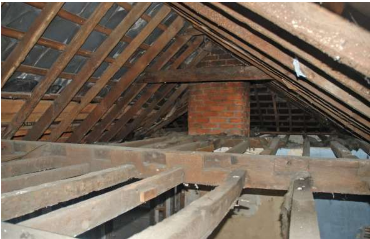
Fig.104: Roof space over room F1, facing WSW towards chimneystack and room F3
