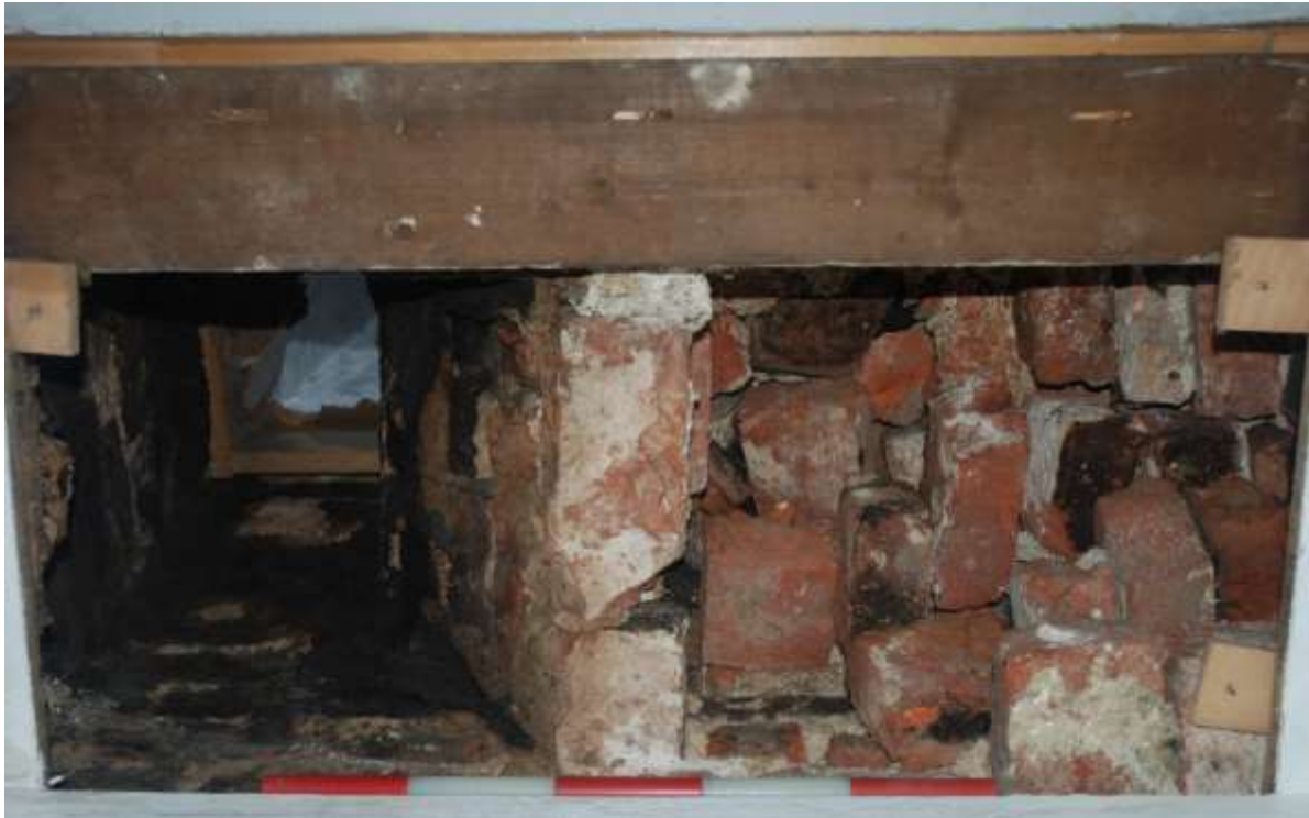
Fig.33: Interior of former flue above fireplace in the northeastern corner of room G1. North to left of frame. 0.50m scale
