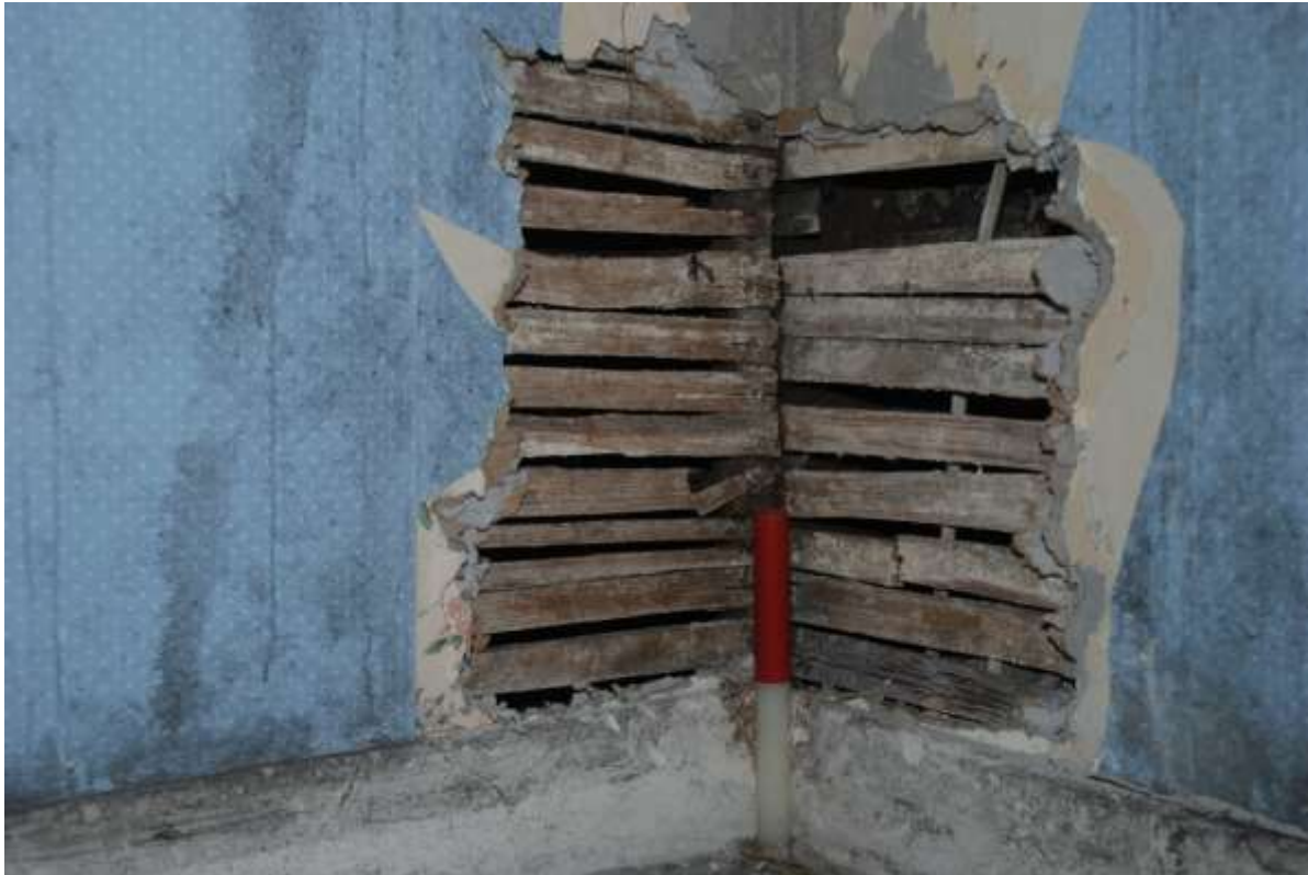
Fig.71: NW corner of room F1, showing the laths abutting, but clearly of one build, 0.20m scale
