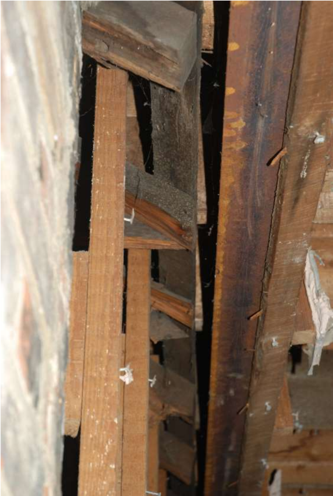
Fig.94: Original roof rafters at rear of property, (room F5), having been cut back to fit RSJ. Looking up from north side of chimneystack
