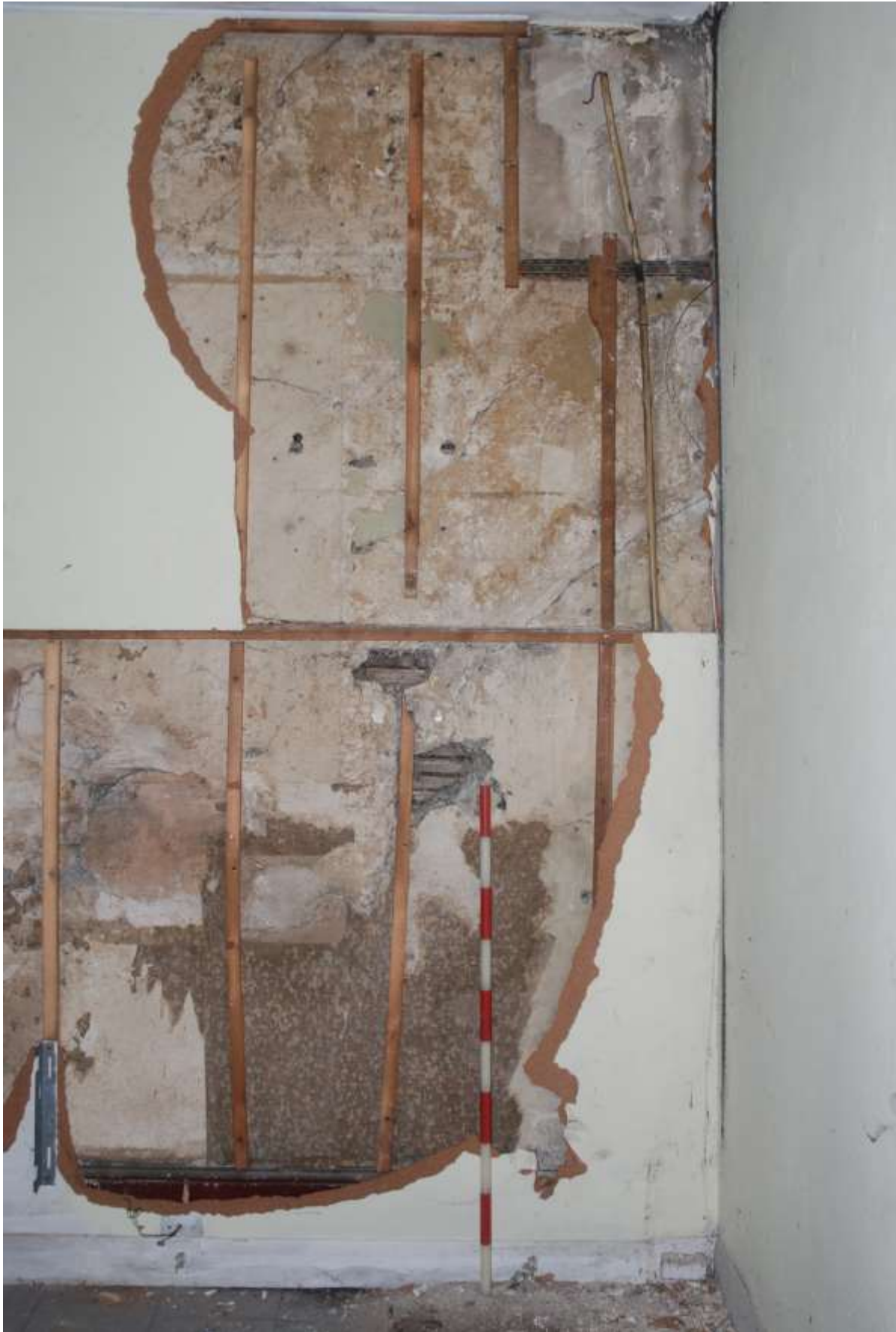
Fig.39: Southwest corner of room G1, facing SSE, 1m scale. Detail of former decorative schemes and lath and plaster construction
