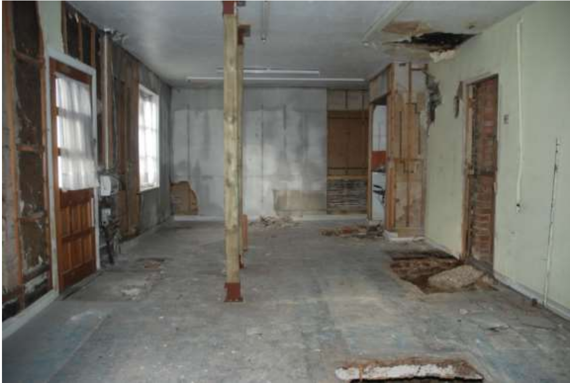
Fig.26: Room G1 facing N, front door to left of frame, holes to cellar in floor
