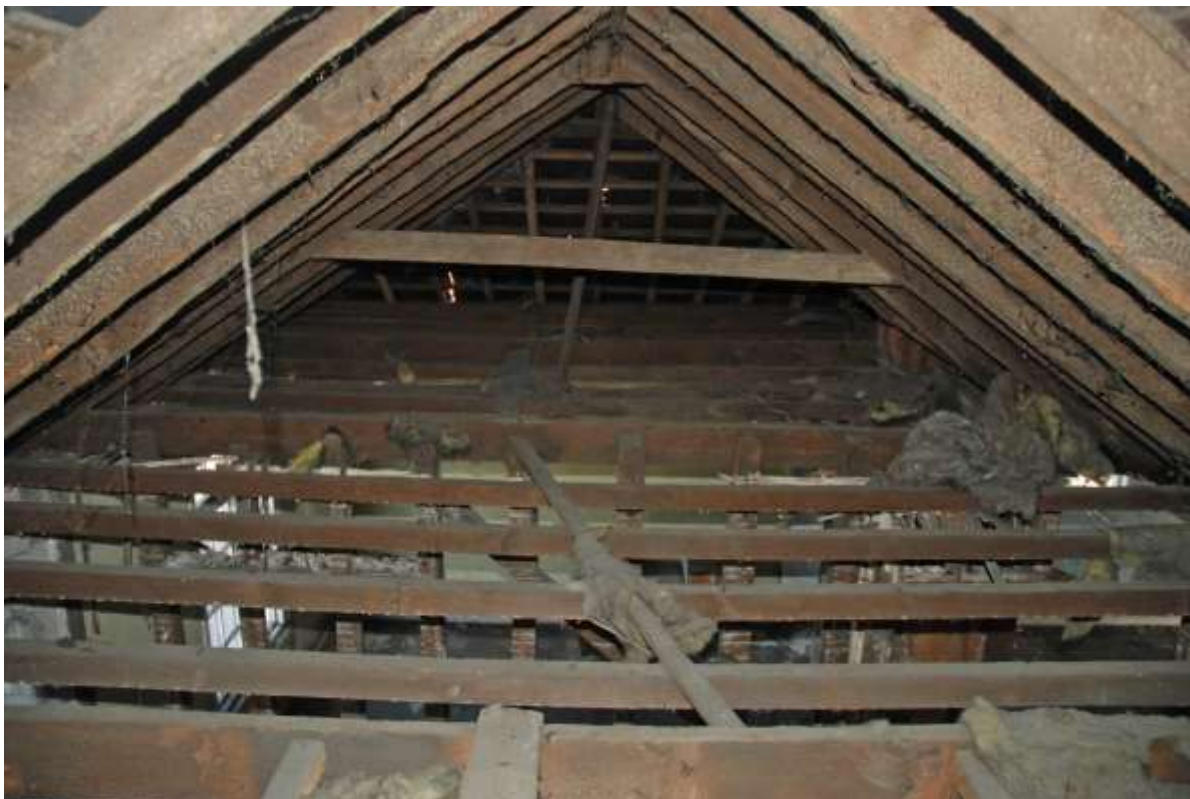
Fig.101: Roof space over room F4 facing N, showing sloping end of original hipped roof line
