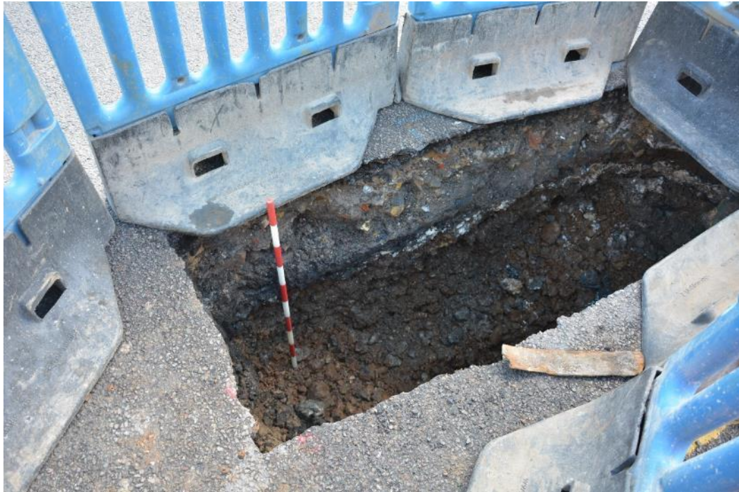
Figure 7: Trench 6. Dark orange gravels (4) can be seen below a thin black lens (3) and rubble abundant road make up (2). Facing SE. Scale 1m.
