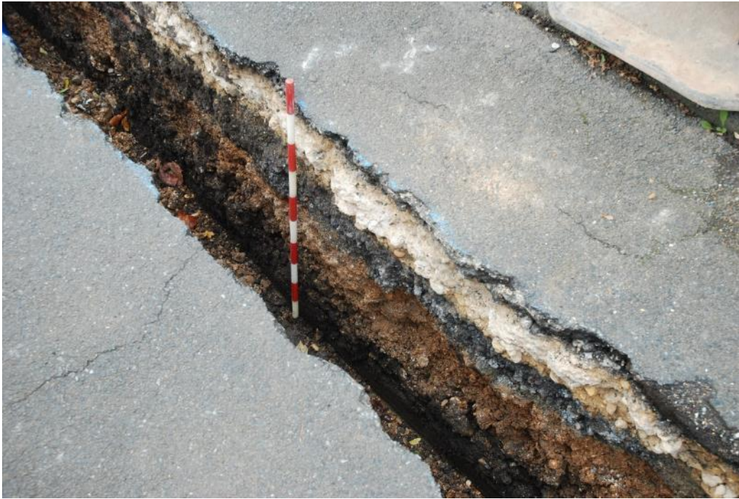
Figure 11: Detail of the concrete bedding layer (5) for the asphalt road surface (1) observed in Trench 8. Facing SW. Scale 1m.
