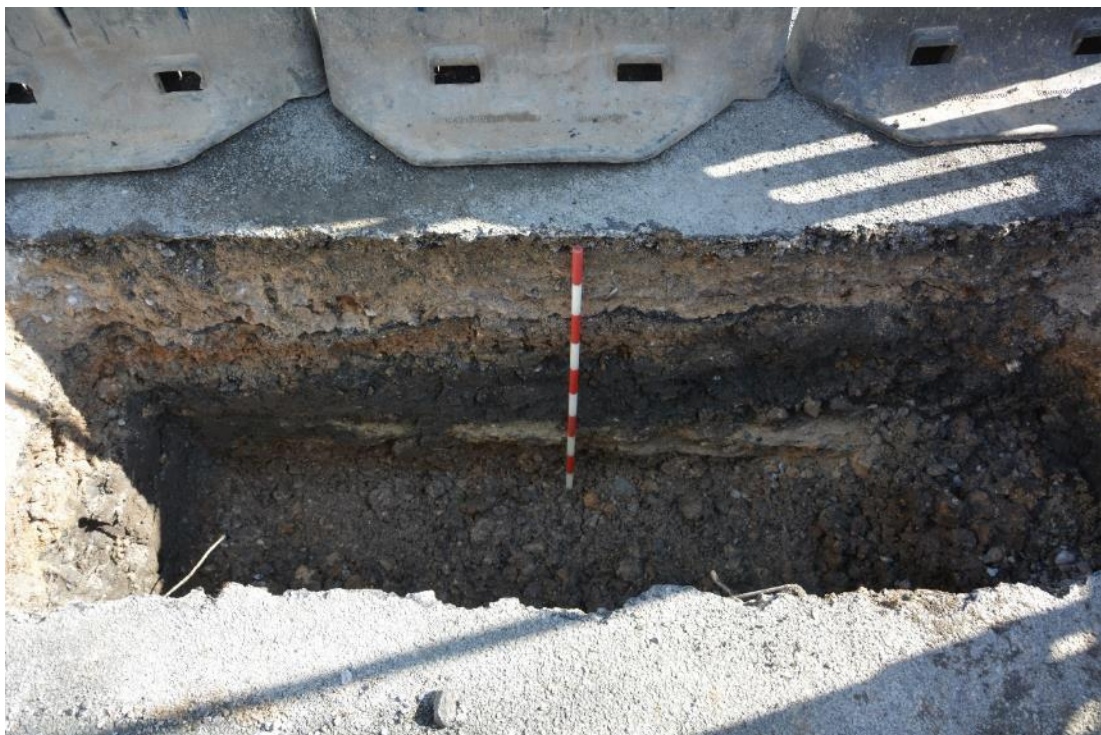
Figure 6: Trench 1. Gravels (3) and (4) below road surface and make up (1) - (2). Facing E. Scale 1m.
