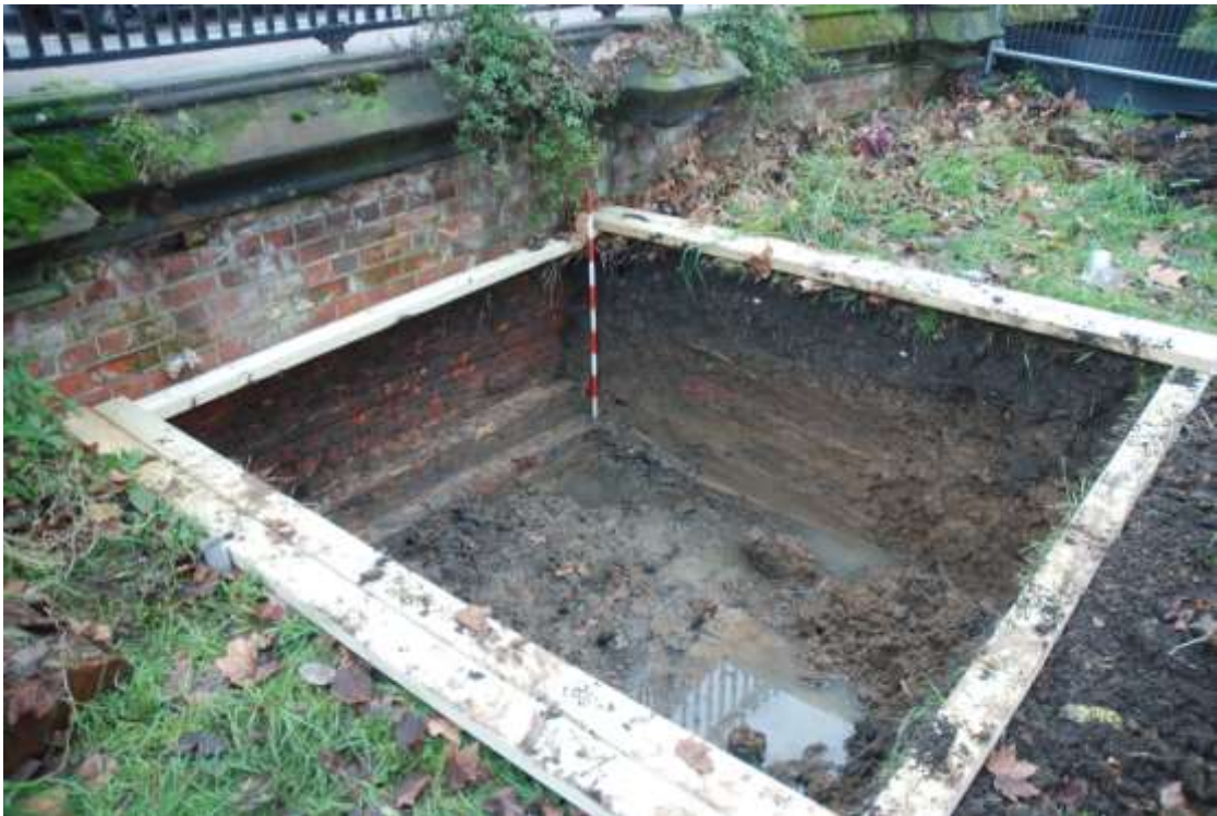
Figure 11: Trench, at a depth of 1.0m. The stepped foundations of the wall can be seen to the left of the scale. Facing S. Scale 1m.
