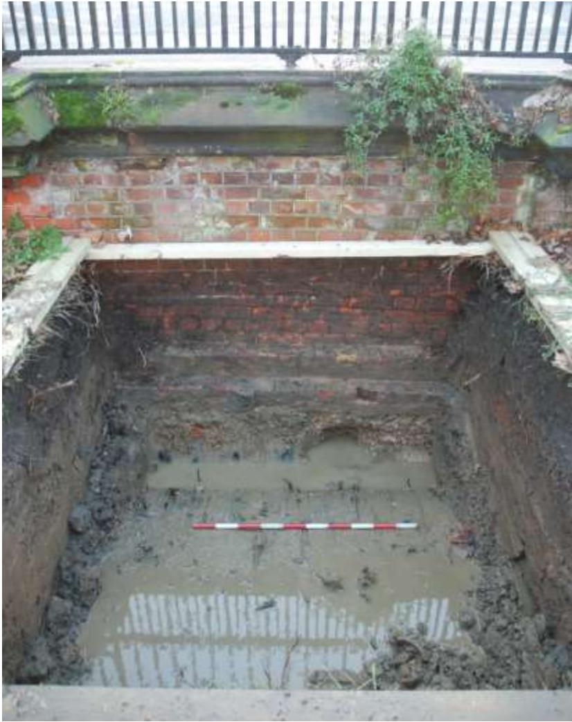
Figure 13: Completed trench, showing foundations of wall [4], water ingress from gravel (5) and natural clay (3). Facing SE. Scale 1m.
