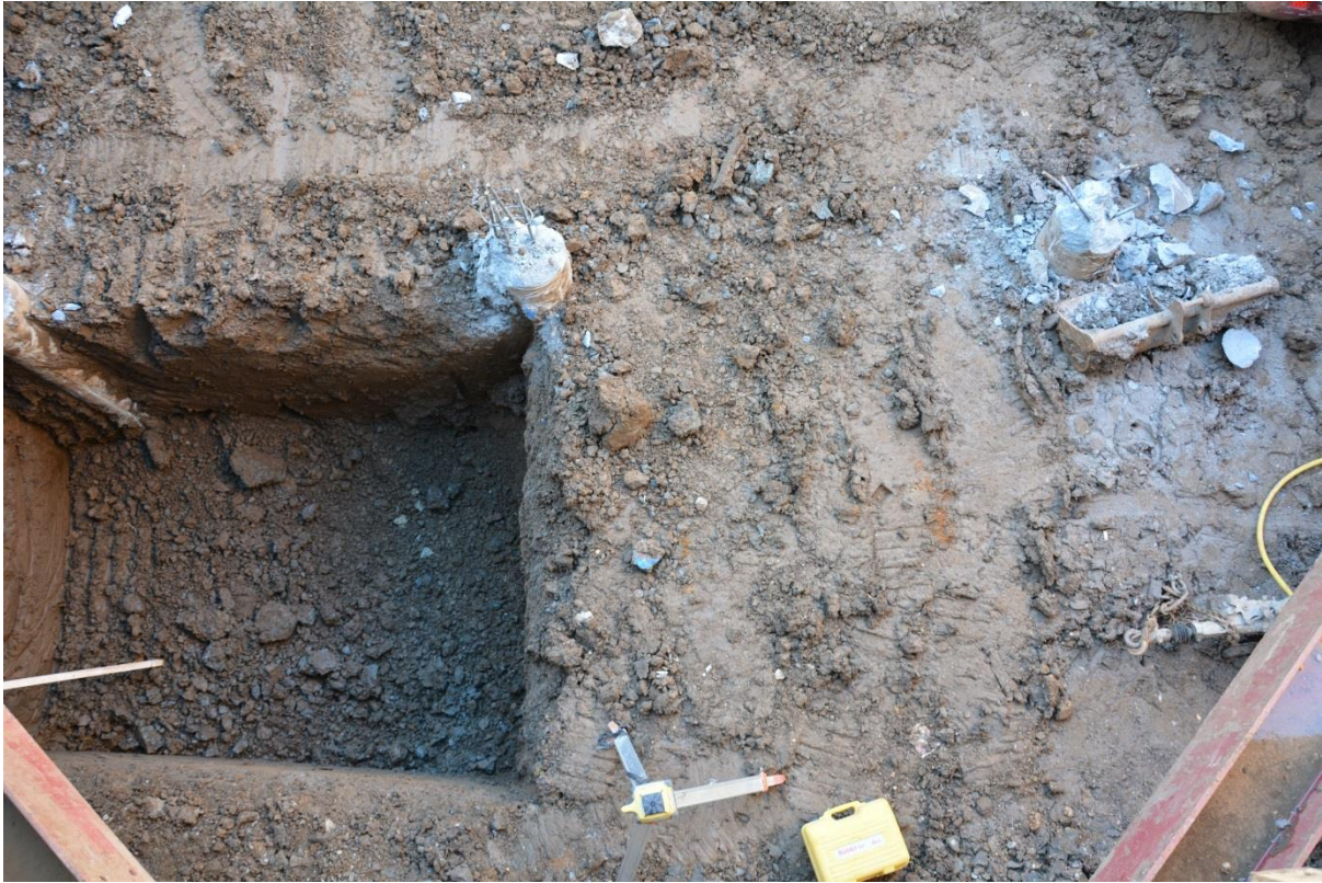
Figure 13: Large hole dug at east end of site. Facing W, no scale
