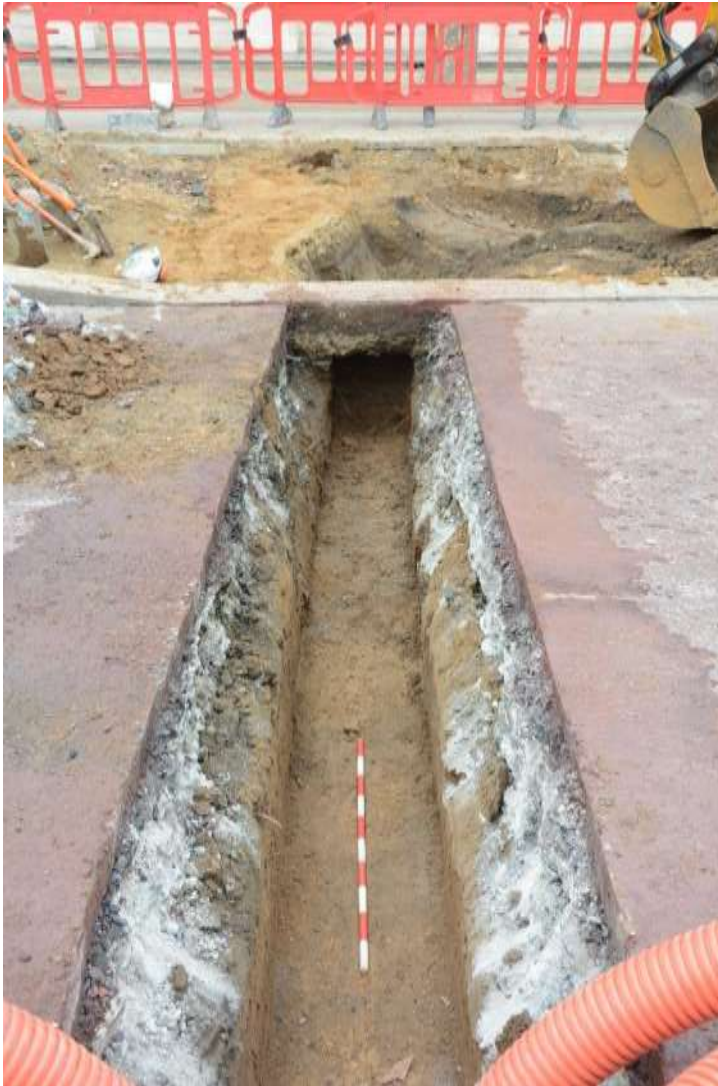
Figure 15: Northwestern end of eastern trench (looking towards Carlton Terrace) showing the groundworks below the road and North Horse Ride. Facing NW. Scale 1m.
