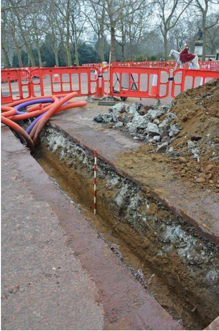
Figure 16: Southeastern end of trench, showing sand below road make-up. Facing S. Scale 1m.
