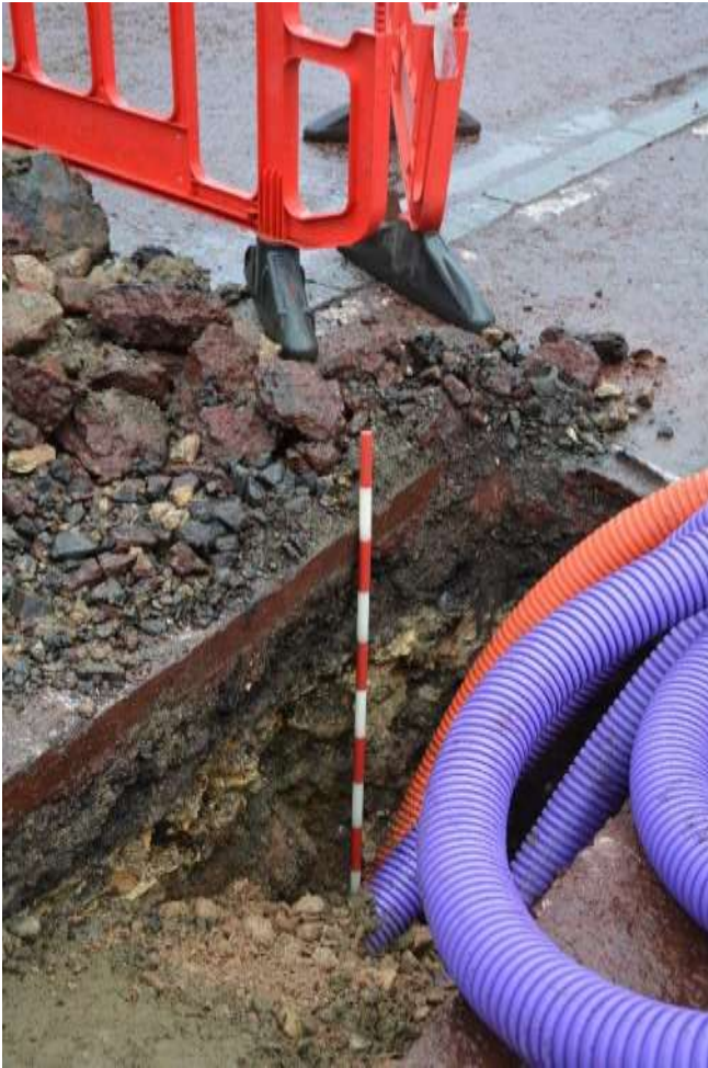
Figure 12: South facing section of east-west trenching across Horse Guards Road, showing post-medieval / modern backfill below modern road make-up layers. Facing NE. Scale 1m.
