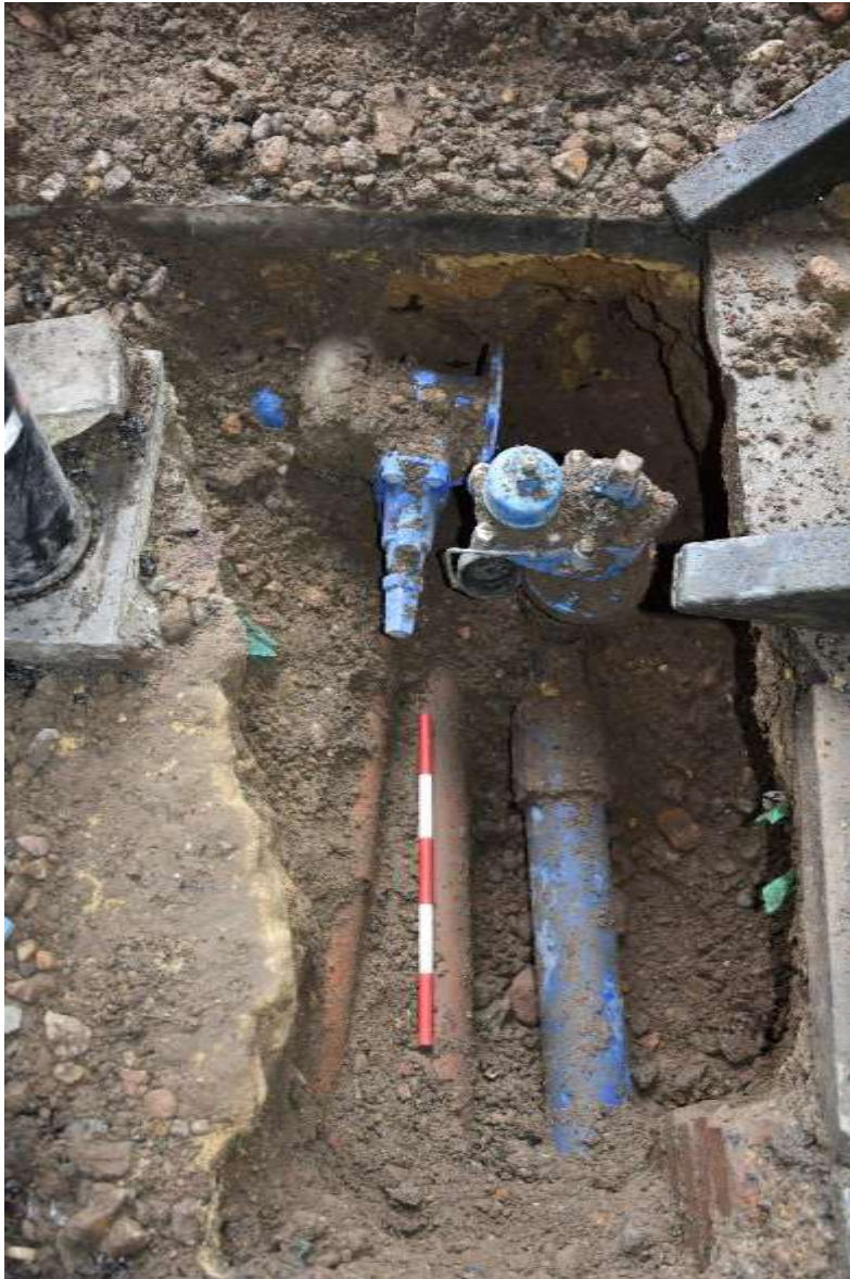
Figure 9: Re-excavated spur, showing TW main and valve and orange coloured services [14] / (15). Facing W. Scale 0.5m.
