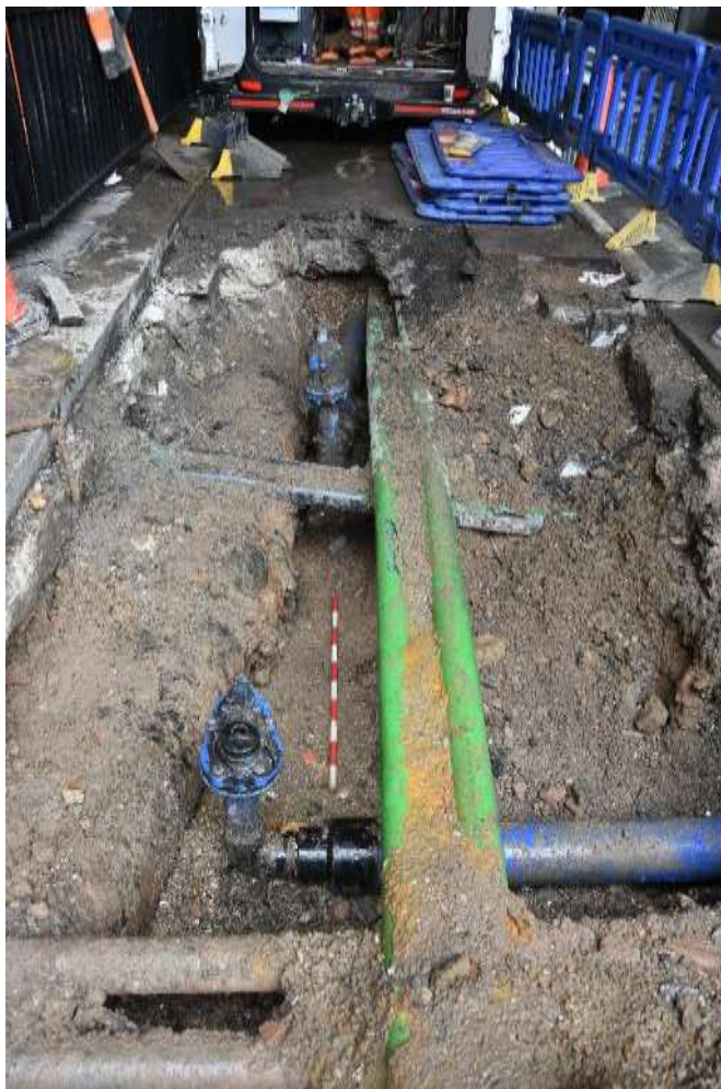
Figure 6: View of the completed trench, showing multiple services cutting made ground. Facing E. Scale 1m.
