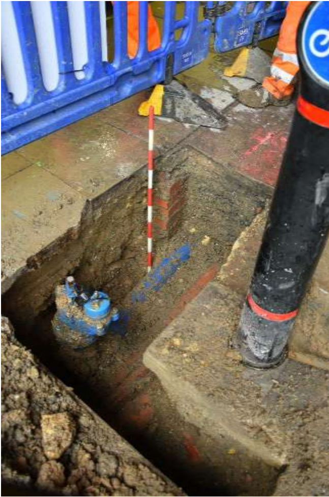
Figure 7: Additional spur on the northern side of the main trench, showing east-west water main and services [14] / (15). Facing approximately NE. Scale 1m.
