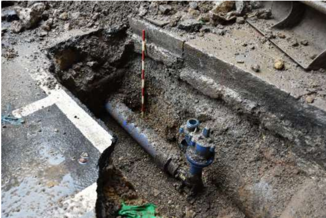
Figure 8: South facing section of trench, showing existing cycle way surface and bedding above made ground. The large gas main [4] / (5) can be seen to the right of frame. Facing NW. Scale 1m.
