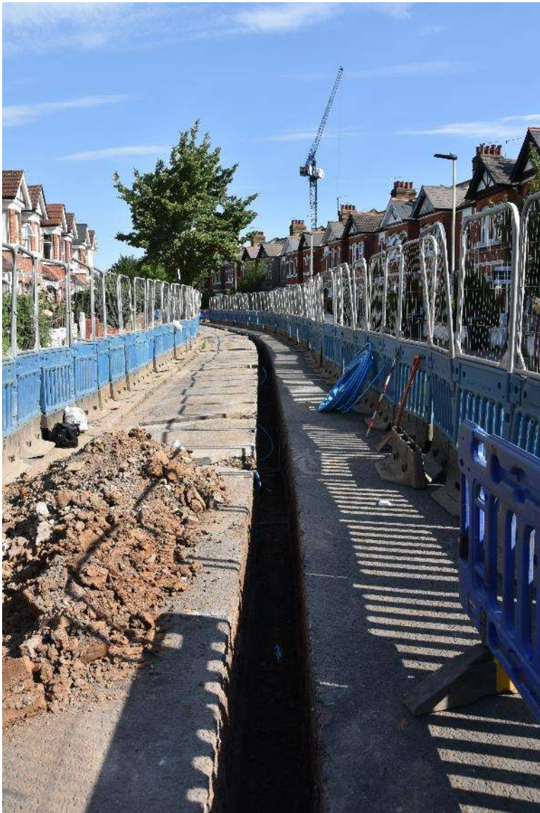
Figure 9: Working shot, showing the main trunk trench with spurs seen to the left of frame. Facing approximately N. No Scale.
