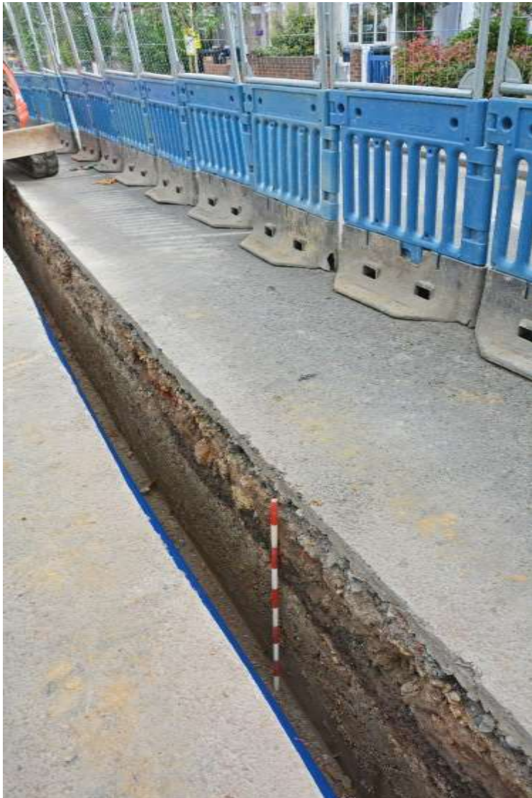
Figure 10: Stratigraphy observed at the southern end of Seaford Road. Approximately 0.4m of post-medieval and modern stratigraphy can be seen above natural clay. Facing NNE-NE. Scale 1m.
