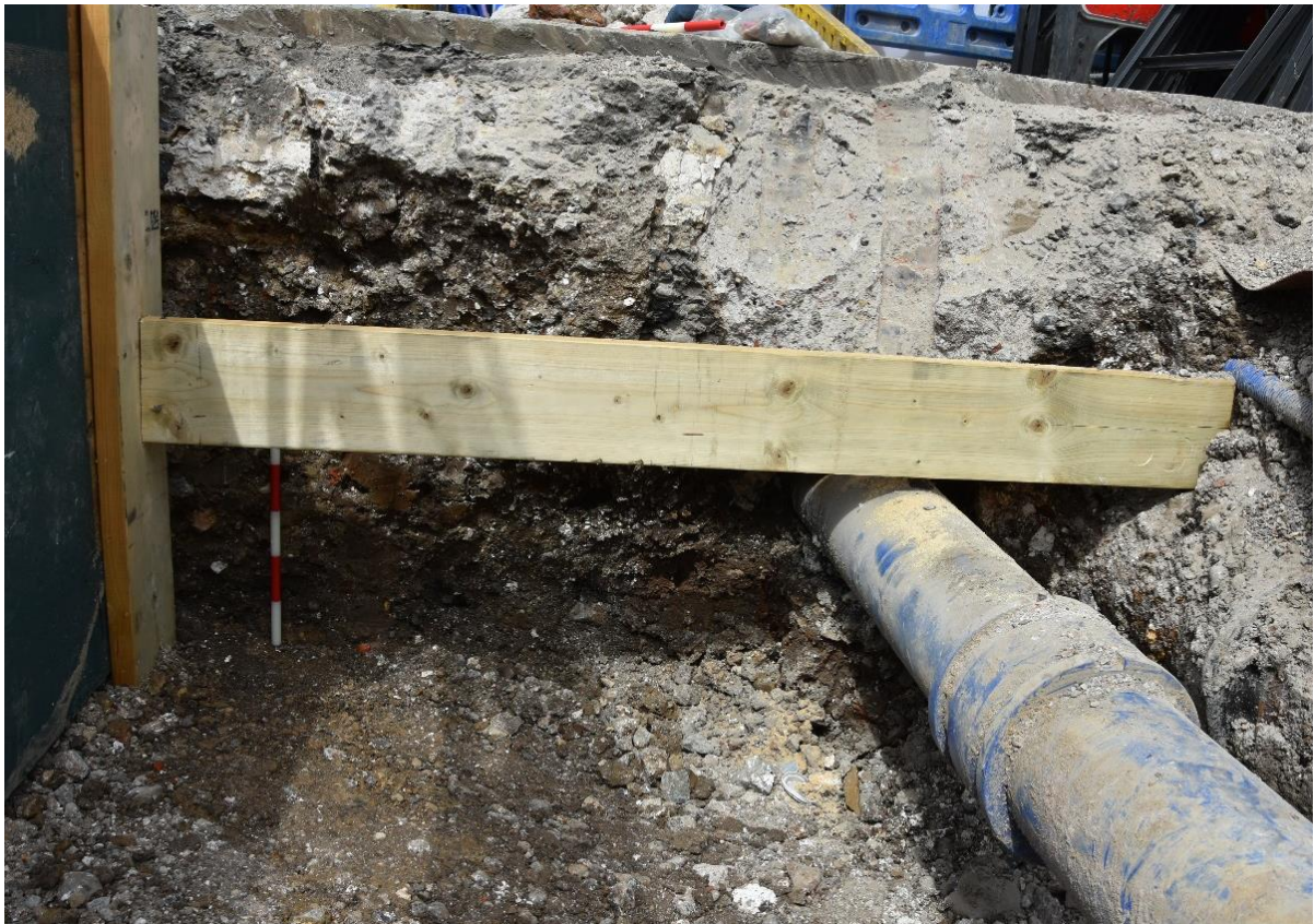
Figure 15: Detail of south-facing section (Section 2), in northern end of trench (0.5m scale); illustrating water main (blue) [11] and unknown service pipe (far right), backfilled with concrete (10), truncating dark layers of made-ground (12), (13), (14) (left)
