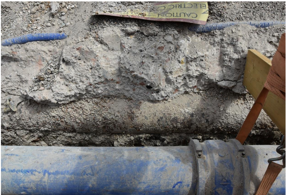
Figure 13: Detail of disturbance caused by water main (below) and unknown service pipe (above), both running N-S, in west-facing section
