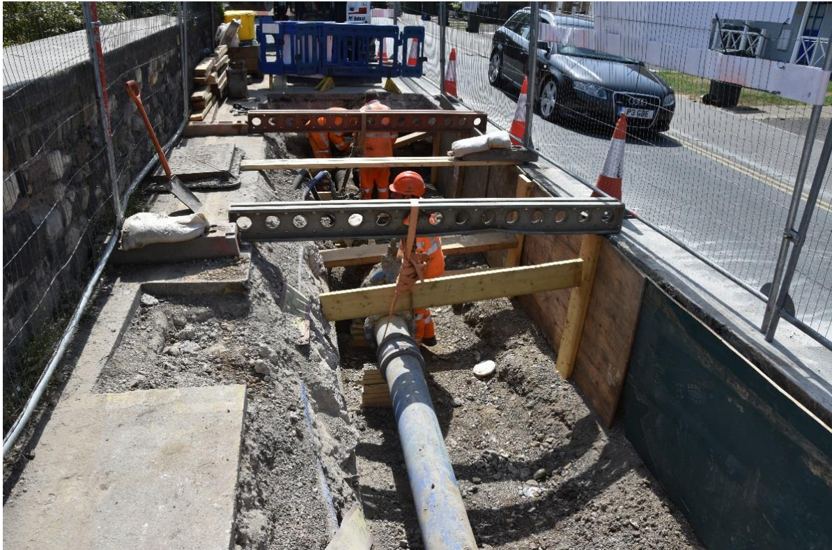
Figure 11: General shot of the excavated trench, facing SW; the water main is shown in the centre of photograph
