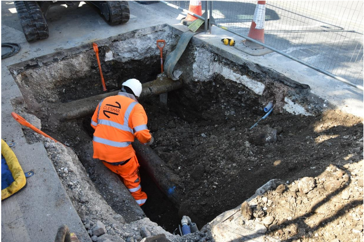
Figure 12: Detail of trench, facing SW, highlighting extensive disturbance caused by modern services
