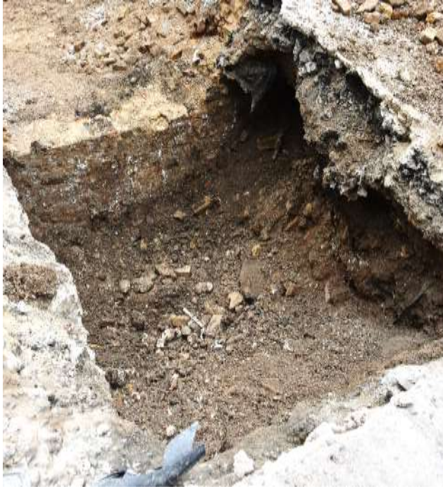
Figure 7: Collapse of south facing section in eastern end of trench with [104] in centre. No scale.
