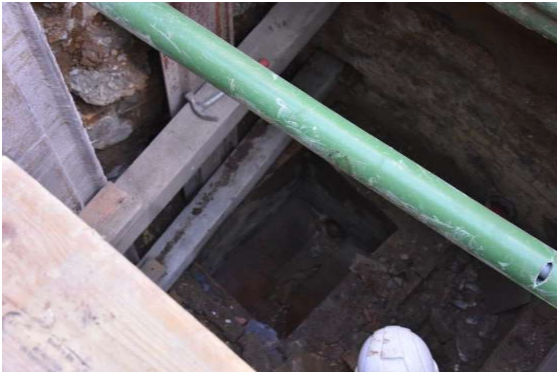
Figure 8: Working shot of the open inspection chamber to the south of the coal cellar [6], as seen from the top of the drop shaft. Facing NW, no scale.
