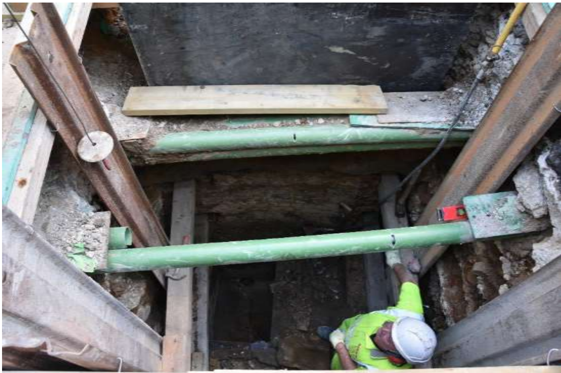
Figure 4: Working shot of completed drop shaft, showing the remains of a brick coal cellar in the northern section and drain in the trench base. Facing N, no scale.
