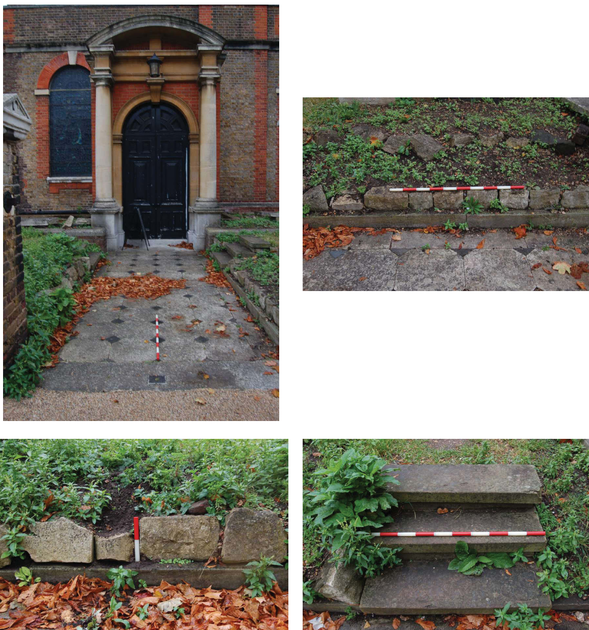
Figure 25: Images of the south porch, retaining walls and steps prior to refurbishment.
