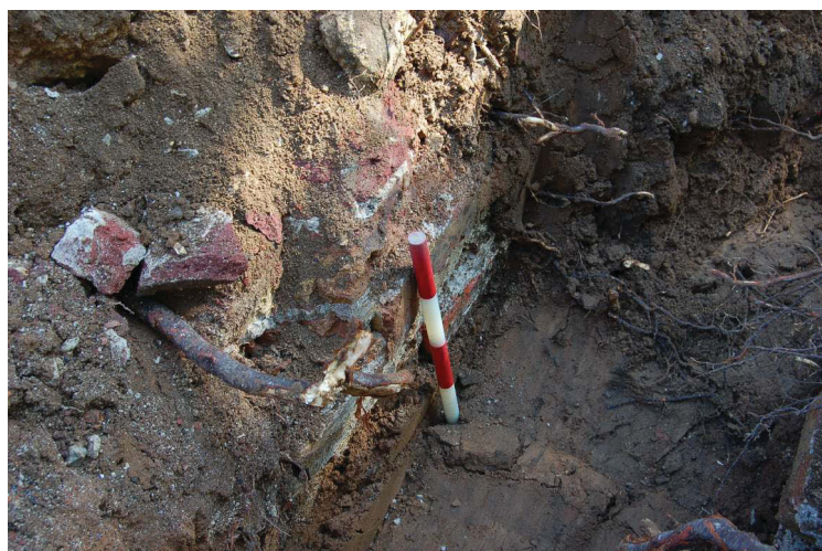
Figure 11: Section of brickwork exposed in Trench A, north facing section, 0.4m scale.
