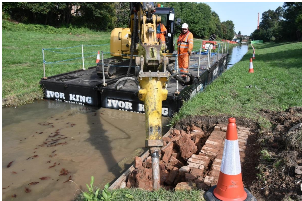
Figure 13: Working shot breaking up the landward section of the east bank. Facing NW, no scale.
