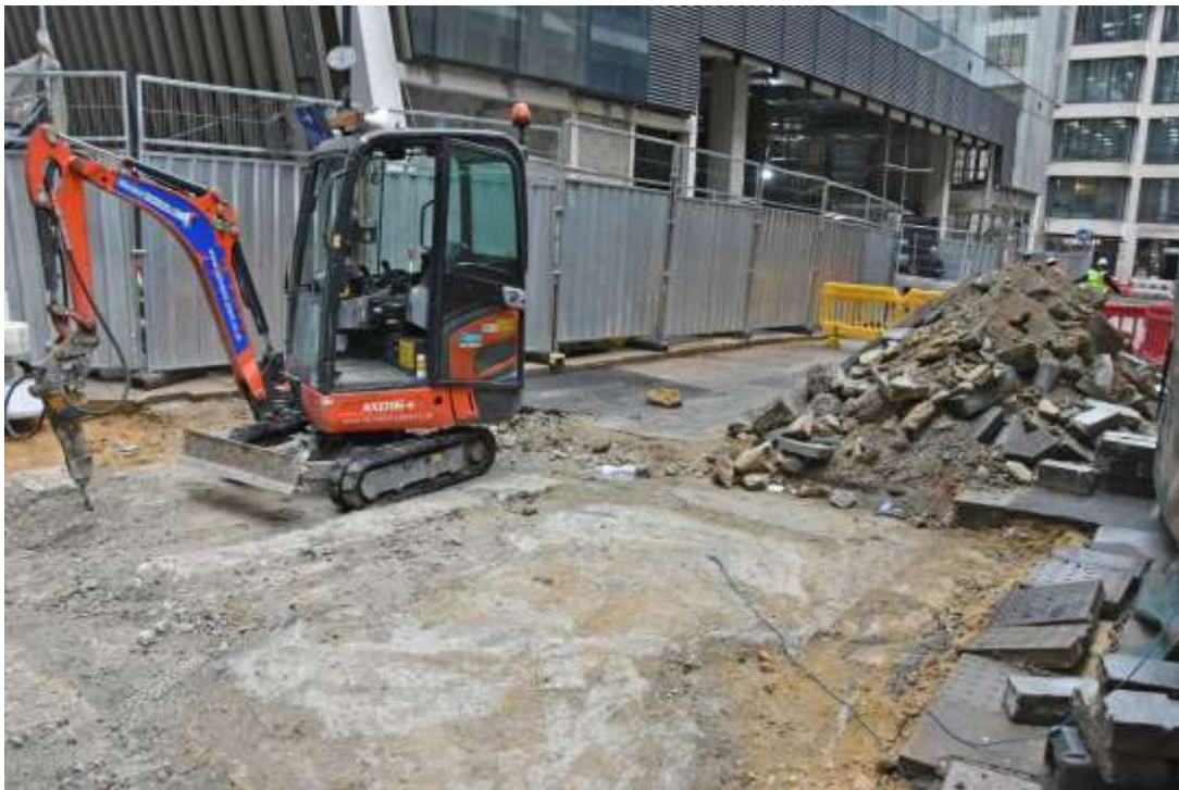
Figure 8: Works area, exposing the concrete (2) following the removal of the tarmac road surface (1). Facing N, looking along Goring Street from Bevis Marks.
