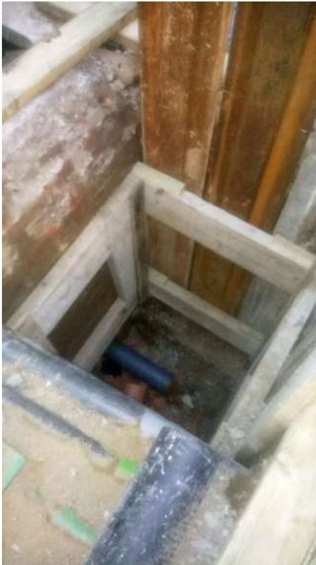
Figure 9: Working shot of dropshaft undertaken at the northeastern end of St Mary Axe. The trench consisted of disturbed made ground, taken to be a result of construction of the existing post-medieval or modern manhole. Facing N.
