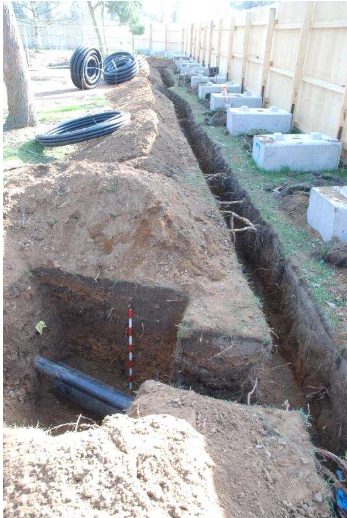
Figure 27: Section of service ducting (Trench 35) excavated along the southern perimeter of the site. Facing E. Scale 1m.
