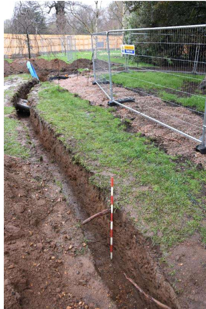
Figure 28: Section of service ducting observed during the completion of Trenches 38-40. Facing W. Scale 1m.
