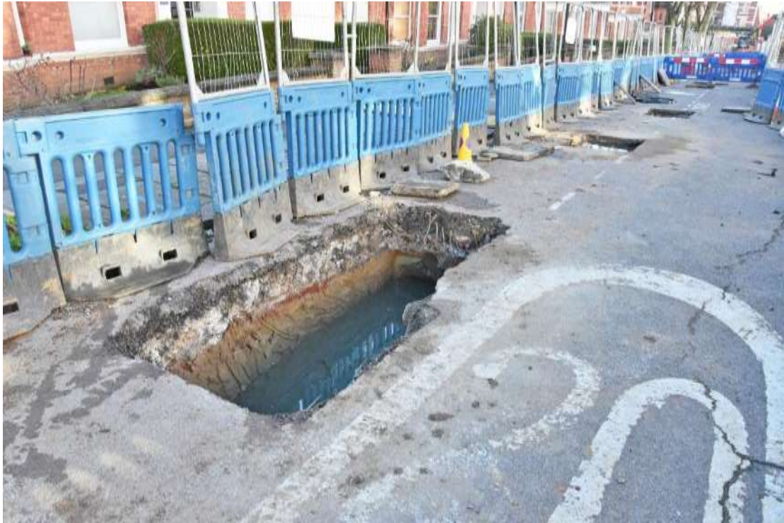
Figure 8: Overview of the works area, showing several flooding trial pits. The same stratigraphy comprising modern made ground over natural London Clay can be seen. Facing approximately S, towards Fortune Green Road.
