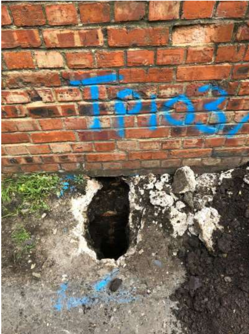
Figure 11: TP103, showing black sandy gravel below the existing concrete. Facing NNE. No scale. Photograph supplied by JOMAS Associated Ltd.
