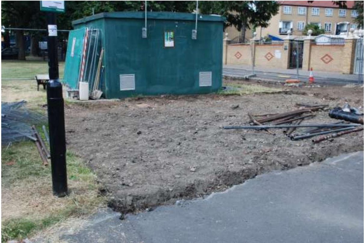
Figure 12: Working shot of the central part of the trench. Facing N. No scale.
