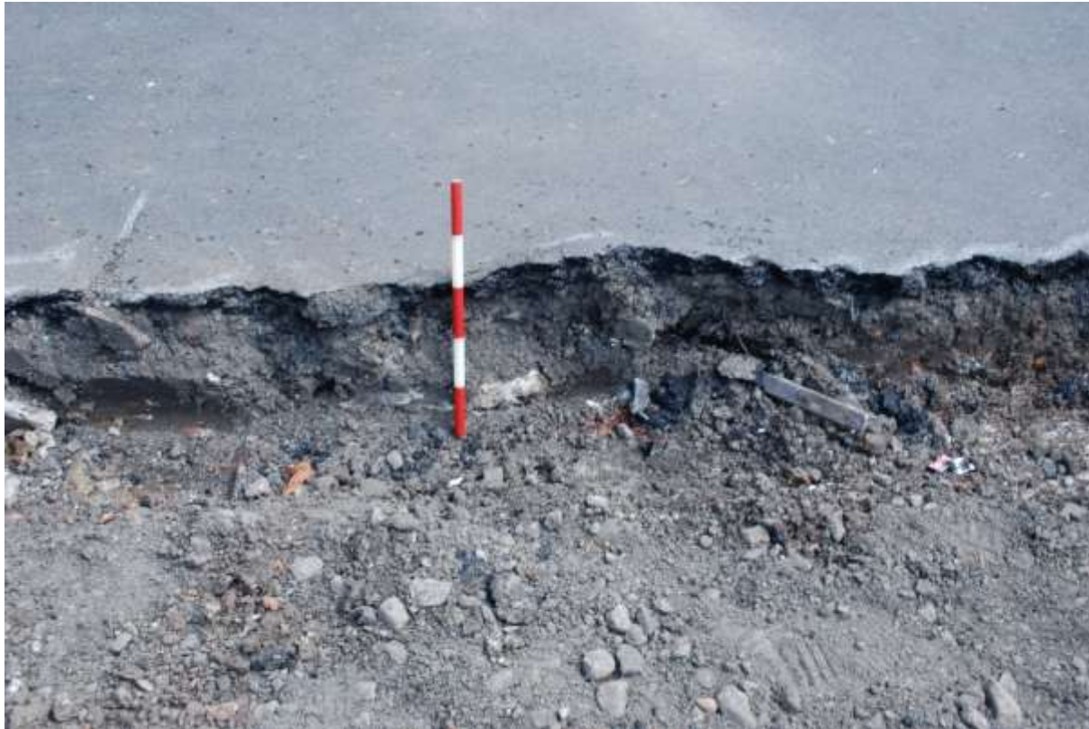
Figure 14: North-west facing section of the central part of the trench through the slot excavated on the south-east side, showing tarmac over made ground. Scale 0.5m.
