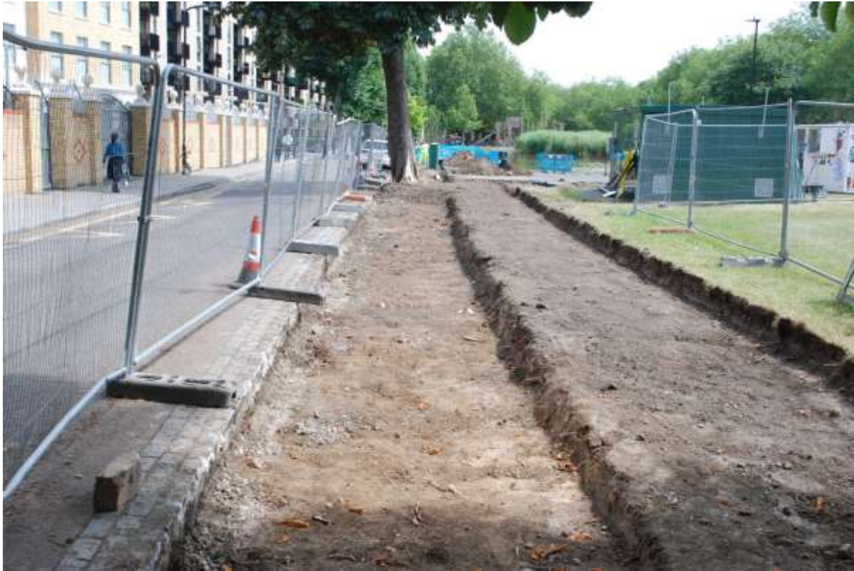
Figure 10: Working shot of the north-west part of the trench. Facing SE. No scale.
