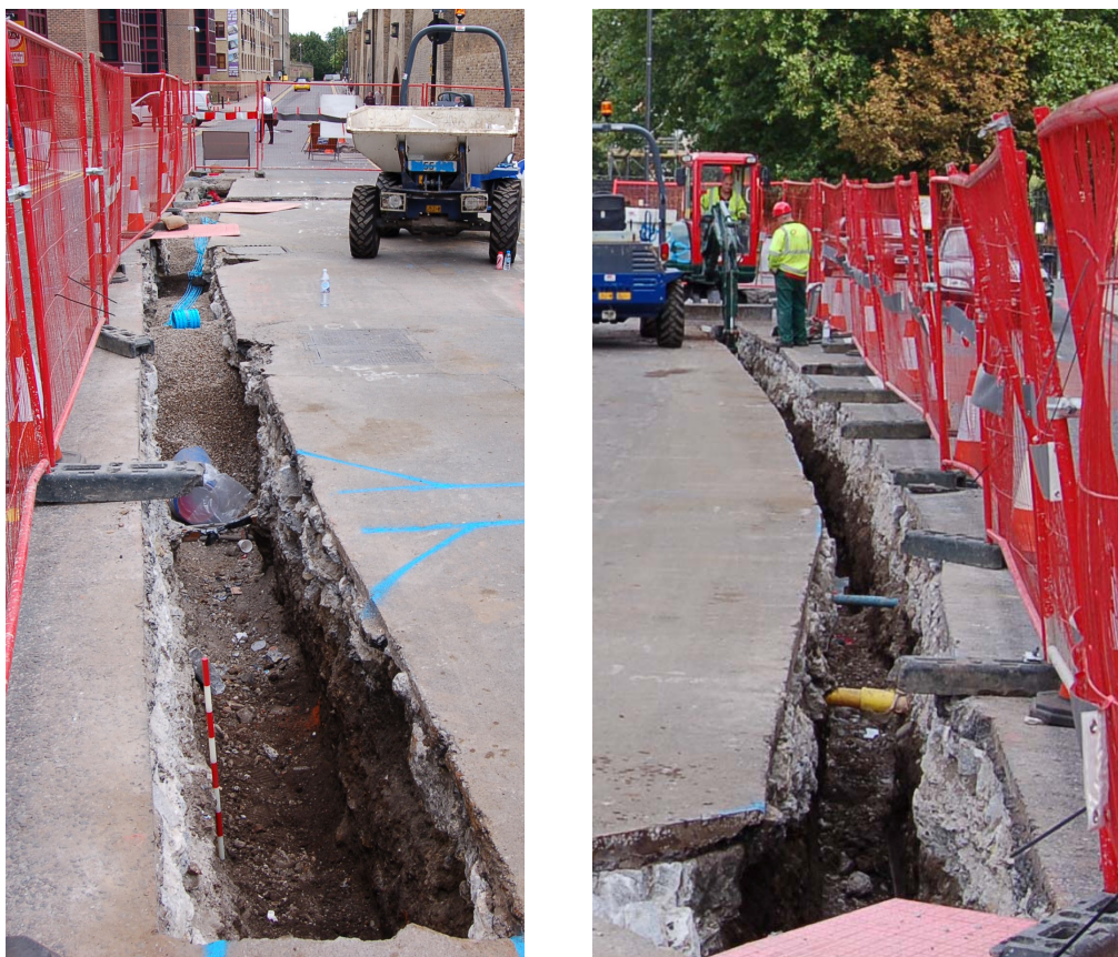
Fig. 16 View of trenching in Wapping Lane. Left: looking south, right: looking north
