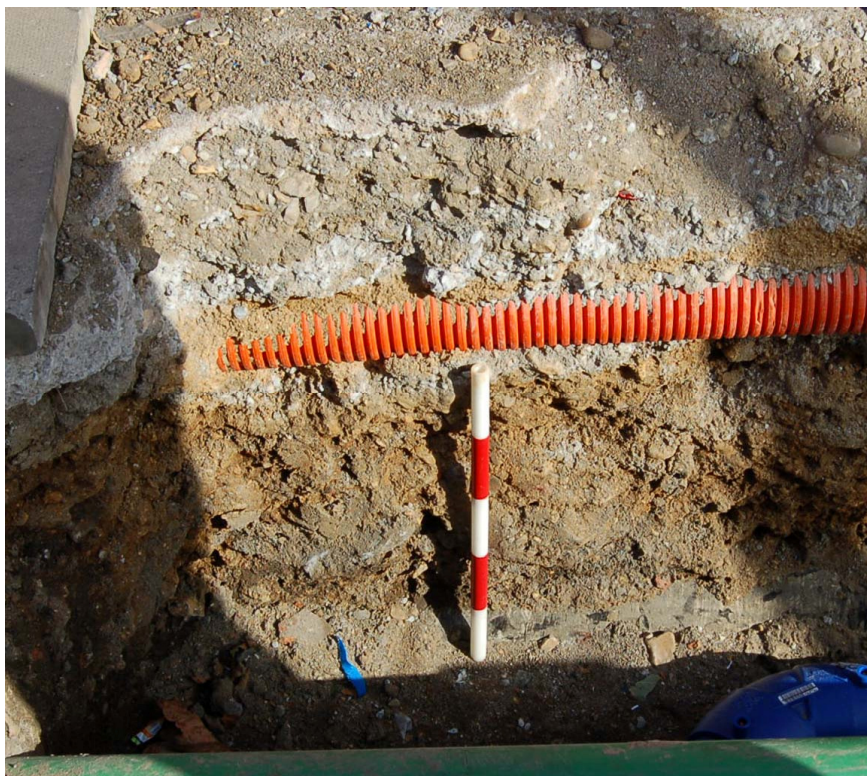
Fig. 14 South facing section on the northern side of The Highway (Scale: 0.5m)
