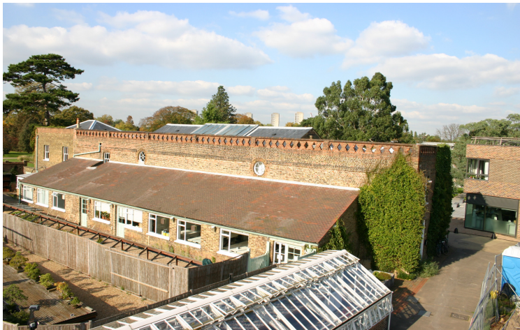
Fig 17 The rear of the Museum No. 2 building, view looking northwest, the red brick parapet has obviously been rebuilt at some stage © John Lonsdale, RBG Kew.
