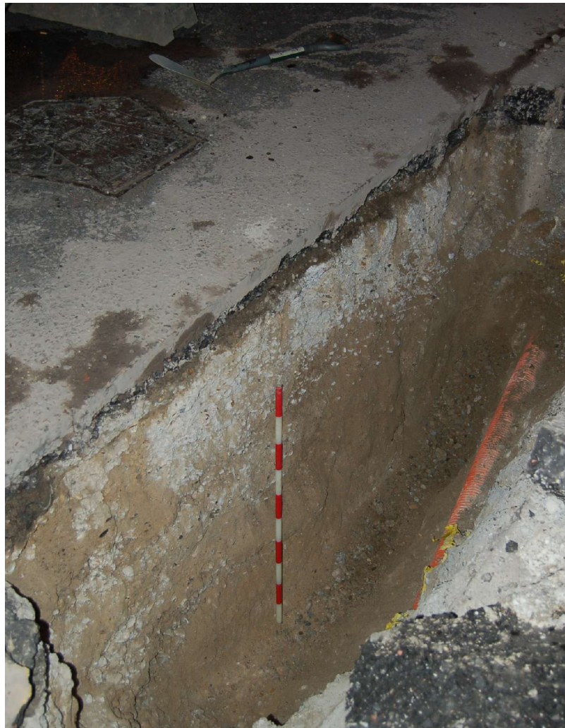
Figure 3: View south of the north-eastern end of Trench 1, showing concrete hardcore beneath the existing tarmac road surface, with an orange-cased cable running approximately parallel.
