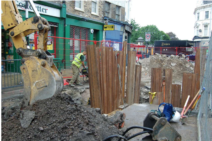
Fig.11 Monitoring groundworks at the northern end of Deptford High Street (just to the north of figure 10), looking north-west.
