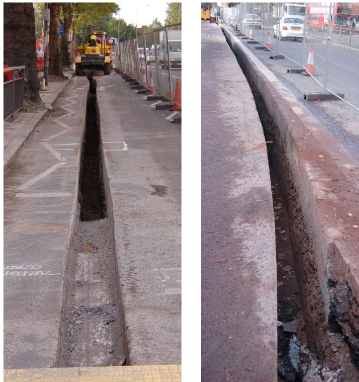
Fig. 12 Views of trenching in the southern carriageway of Creek Road. Looking west.
