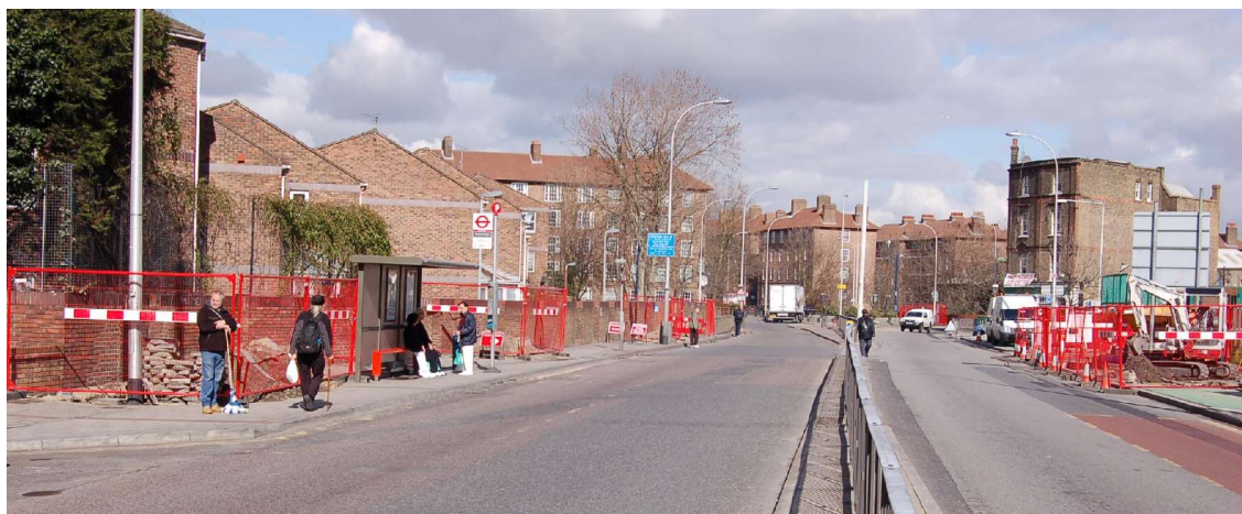
Fig. 4 General shot of groundworks on either side of the Deptford Church Street carriageway; the 100m long trench to the east having been partly reinstated by the time this photograph was taken. Looking north towards the roundabout and junction with Creekside/ Reginald Road.
