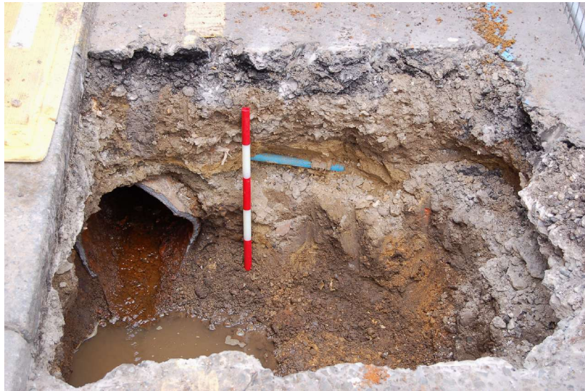
Fig. 7 Pit in the western carriageway outside No. 157 Deptford High Street, showing road make-up, made ground deposits and (to left of the 0.5m scale) the former cast iron water mains now cut and awaiting insertion of the new pipe.
