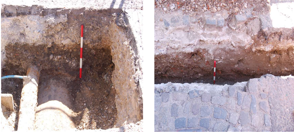
Fig. 9 Left : pit in the eastern carriageway outside No. 200 Deptford High Street, with a very large pipe visible at the base of the trench, and right : a narrow trench to the north dug eastwards into Lamerton Street.
