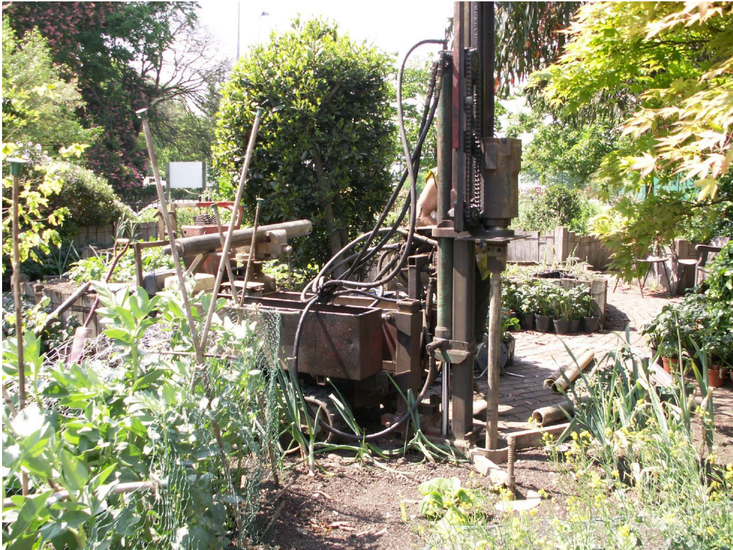
Figure 9 General view showing the extraction of window samples in the centre of the site (WS 4).
