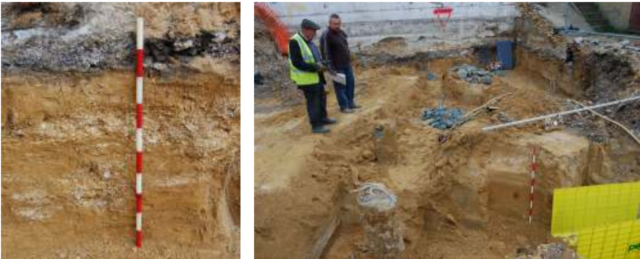
Figure 15 Left: the northwest facing section. Right: The groundworks in the centre of the site, at the eastern boundary looking approximately east
