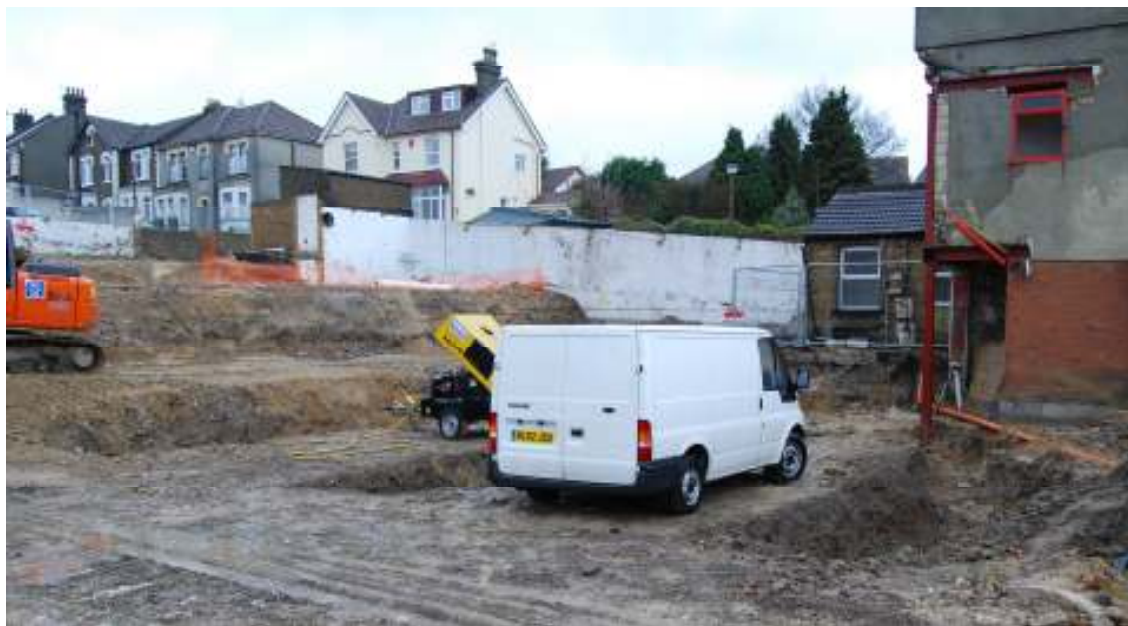
Figure 14 View looking north over trenches 4,5 and 6 (numbered right to left in the photograph)
