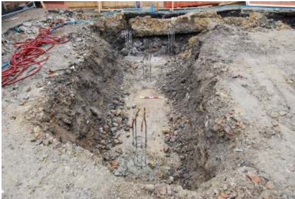
Figure 9 View of trench 1 in the southwestern quadrant of the site, looking southwest
