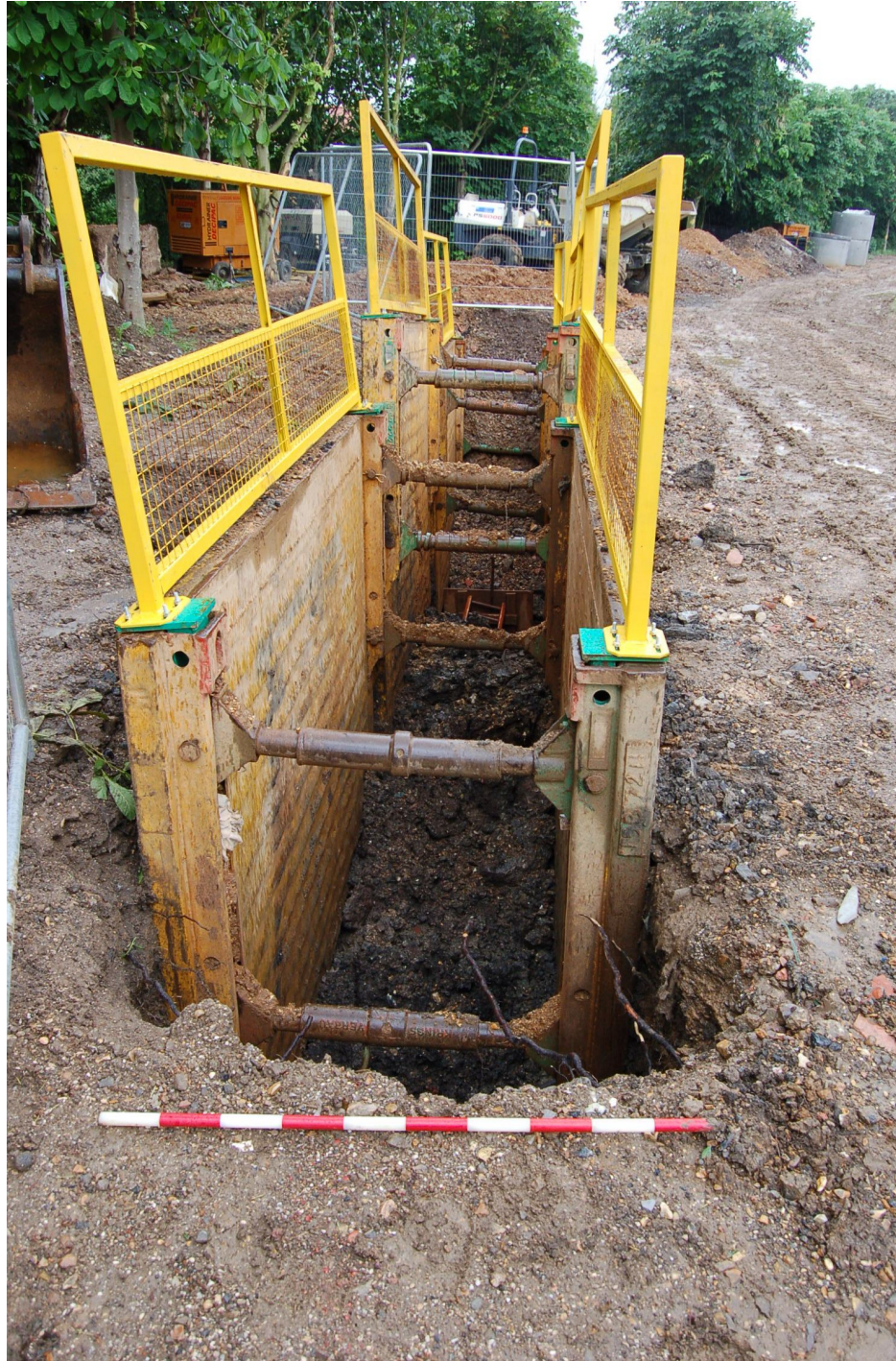
Fig 9: Area of open cut trenching between manhole No.5 and 6 from the northwest.
