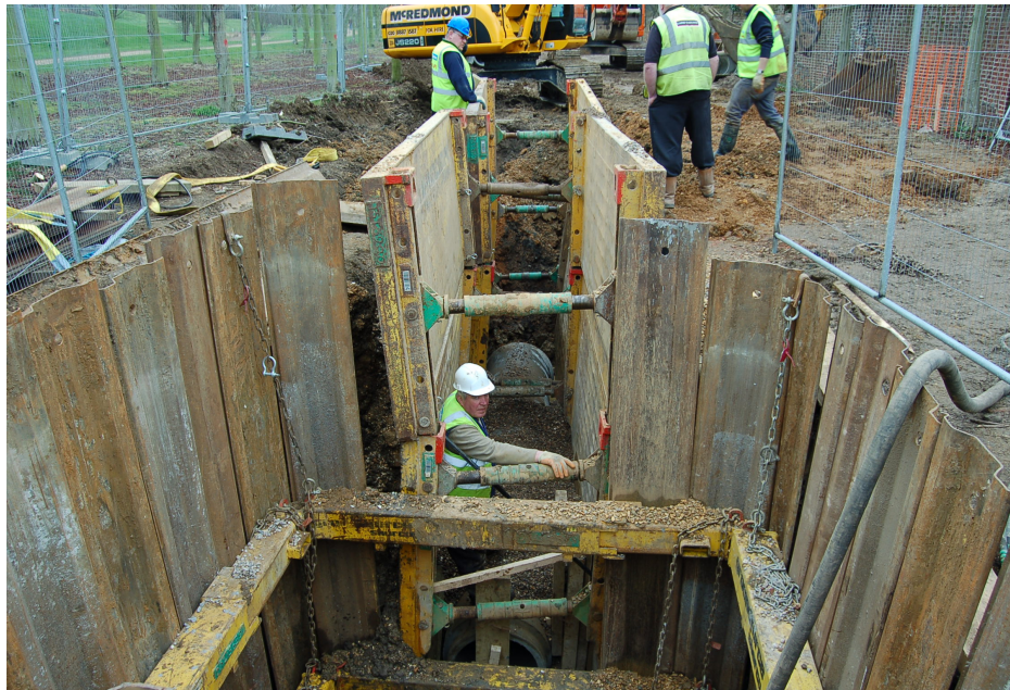
Fig 6: Two trench boxes north of manhole No.10 with the shored up manhole trench in the foreground.
