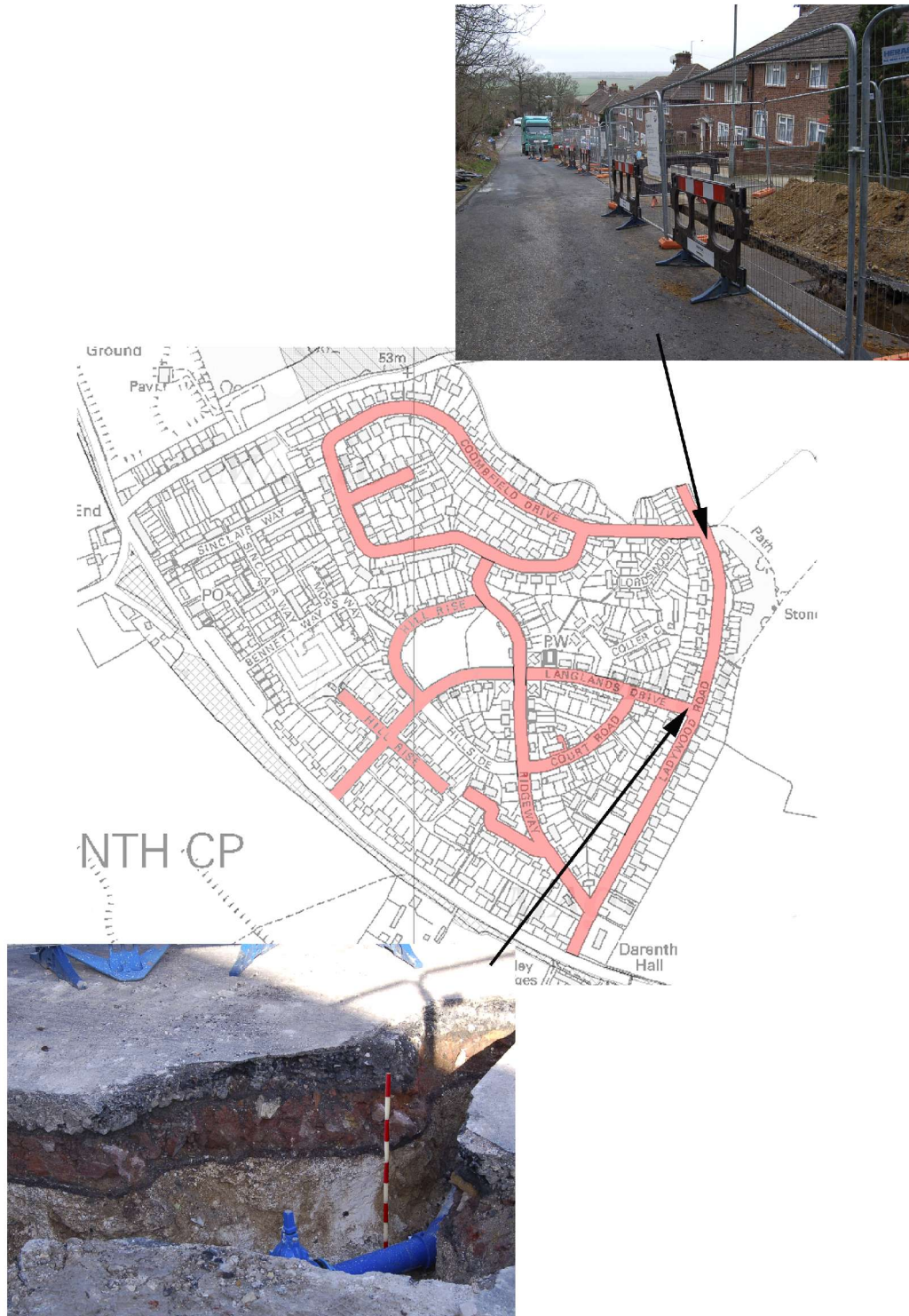
Fig. 6 Views of trenching on Ladywood Road, on the east side of the Darenth area housing estate, with locations marked on the enlarged Ordnance Survey
