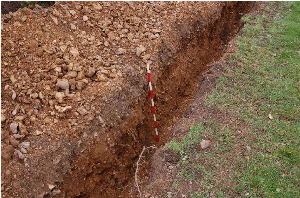
Fig. 9 Views of the first trench monitored in Green Street Green, on the south side of the road and just east of the junction with St. Margaret's Road (1.0m scale)
