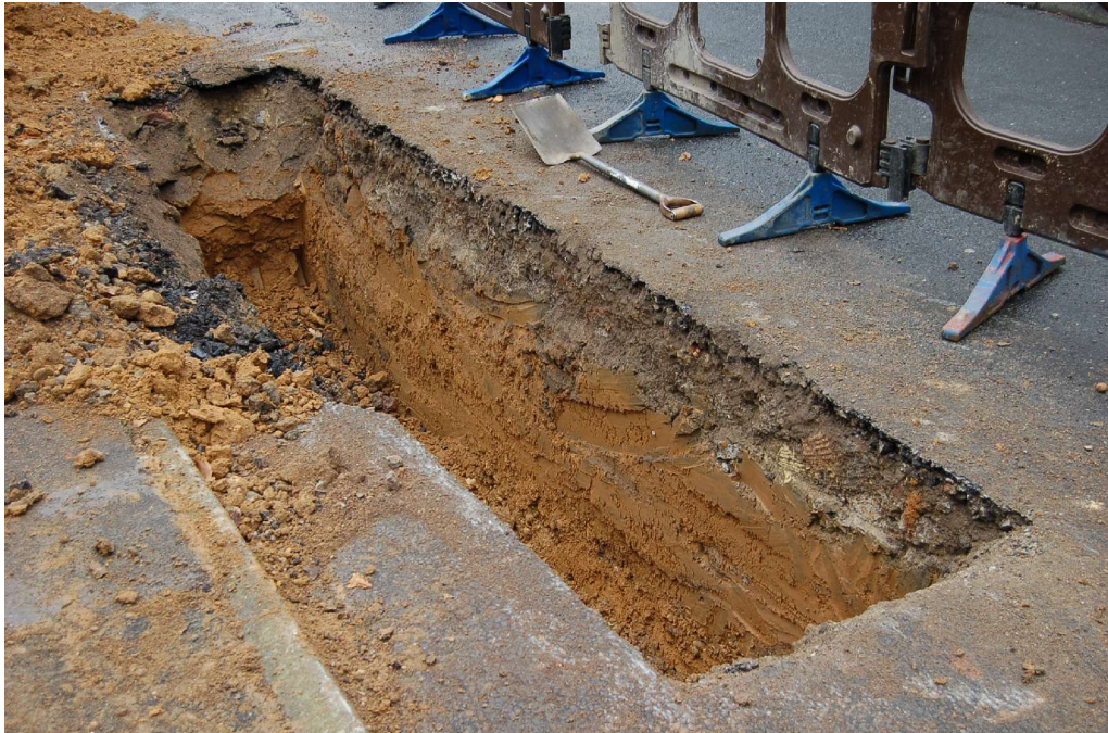
Fig. 5 Further view in Coombfield Drive, showing the natural Thanet Sand deposit directly below modern road make-up
