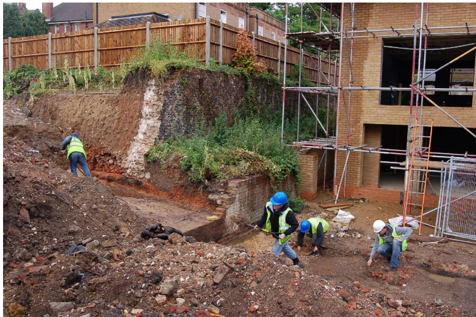
Figure 19: Working shot of Trenches 1 and 5 showing the listed wall [547] extending west behind residential block B.
