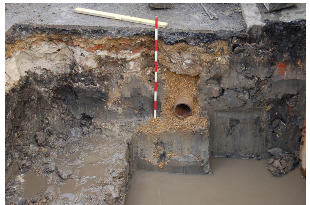
Fig 7: The west-facing section showing the storm water drain and associated sandy fill, cut into the backfill of the larger and much deeper trunk main (scale 1m).
