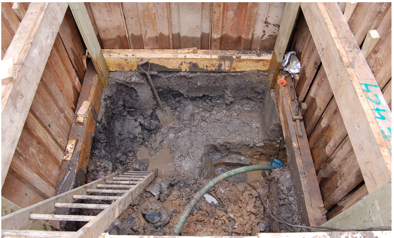
Fig 8: The trench after initially exposing the water main, seen here to the right of the picture.
