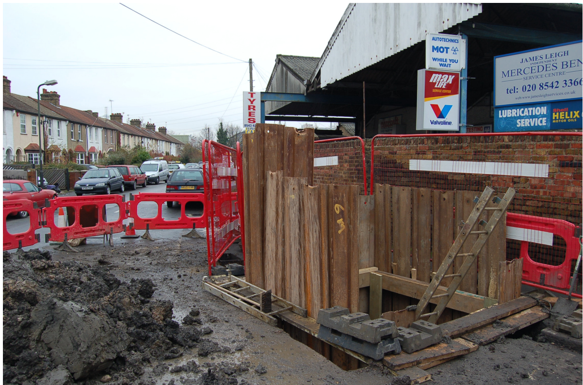
Fig 5: View looking east along the south side of Station Road, with the groundworks in the foreground.
