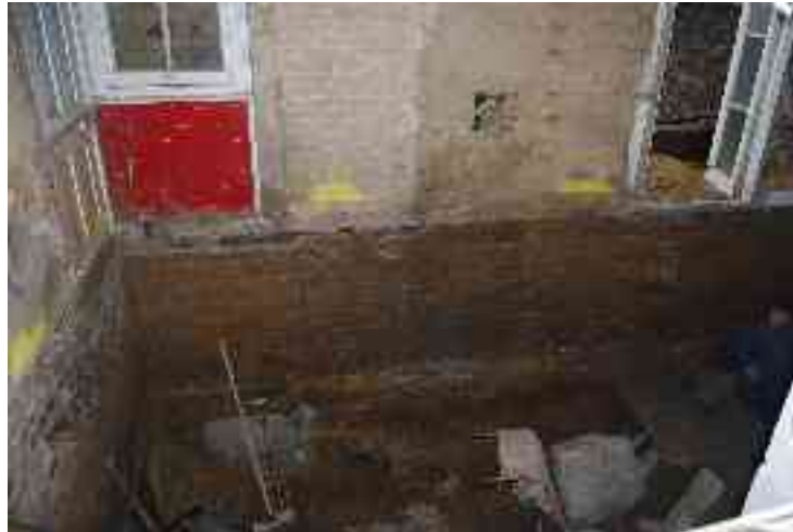
Figure 18: The rear wall of the back room following further ground reduction: the foundations of the wall overlie the rubble base and truncate the natural gravels beneath.
