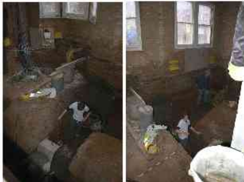
Figures 15 and 16: Inside the front wall of the property prior to further groundworks ( 1m scale ).
