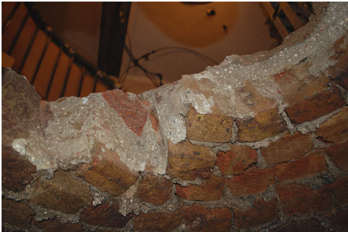
Fig 20 Detail of the brick and mortar construction of the crown of the cistern.
