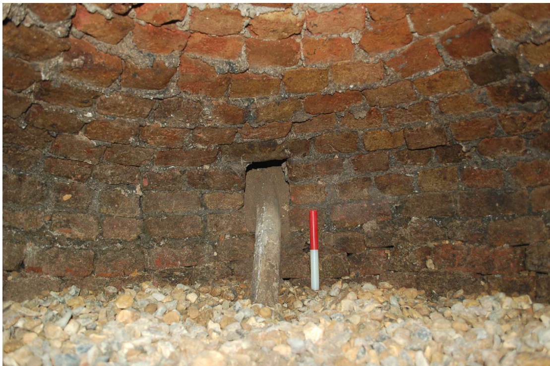
Fig 19 The lead pipe still surviving inside the cistern/well feature. The lead pipe was made in a cast and a mould mark is evident on the pipe (to the left on Fig 18). Lead pipes were first cast c 1539 using a technique devised by Robert Brocke. The lead pipe measured 2½ inches or possibly 3 inches in diameter (7cm). It is reported that the deep end of the lead pipe had been perforated ( pers comm. Stephen Gray, Weldon Walshe). This also seems to suggest that the feature was not a dewatering device or cesspit, but that water was drawn up through the cistern and the perforations acted to filter the incoming water
