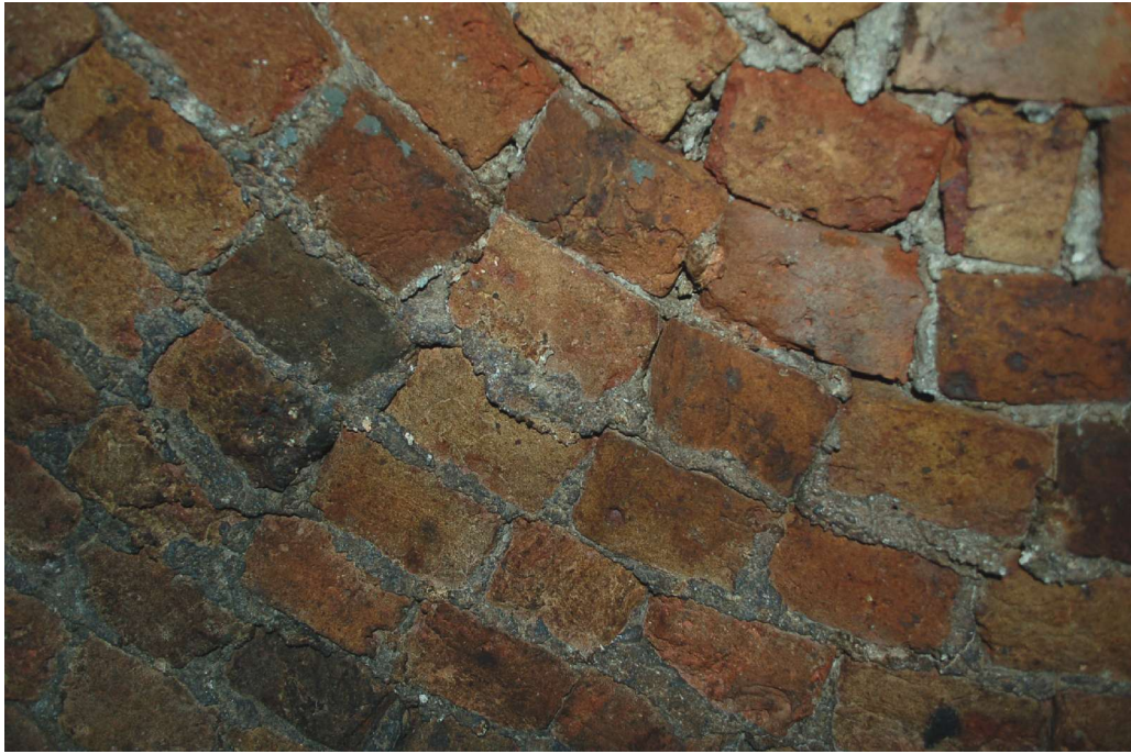
Fig 17 The dome or crown of the cistern was obviously completed externally using an internal timber former or falsework. This is evident in the way the mortar has slipped through the brickwork and hangs in small droplets inside. During construction, it would not have been possible to reach inside to finish the internal pointing (even through the hole for the crown plate) and this would not have been attempted - while the mortar was still wet - for fear of collapsing the structure and of course, it was impossible to fully reach or remove the mortar droplets once they had set. There was no surviving evidence of the timber former used for the construction of the crown.
