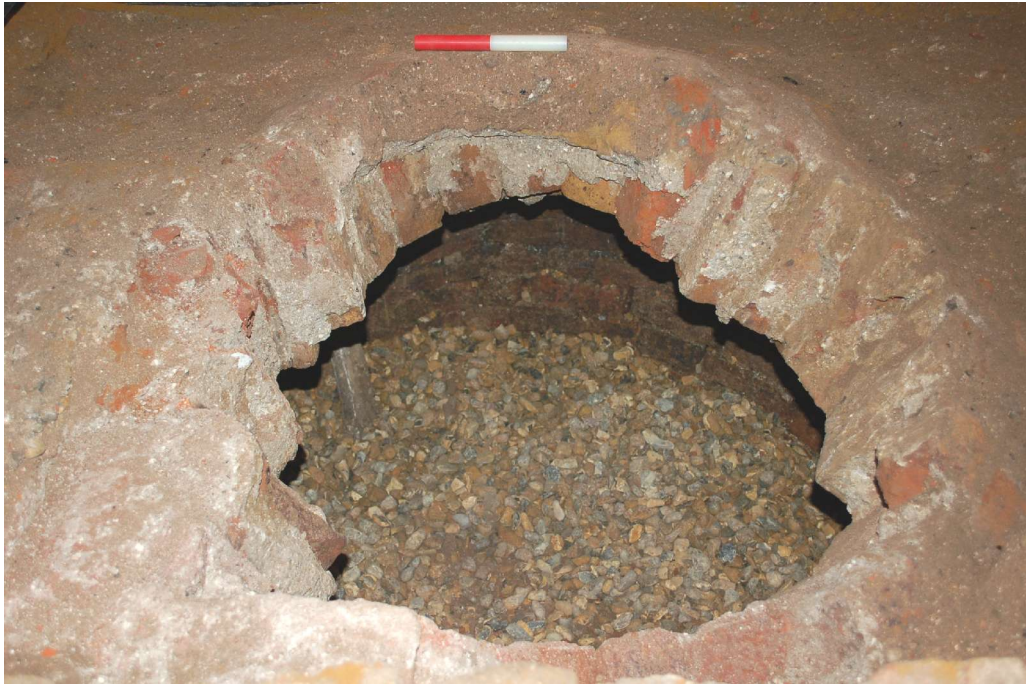
Fig 15 The domed cistern, looking east and internally into the well, which has been backfilled with pebbles for health and safety purposes. The lead pipe can just be seen to the inside the feature on the left-hand side.
