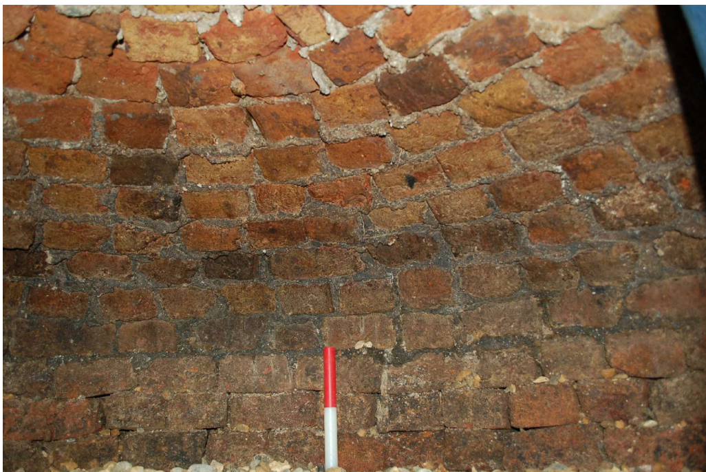
Fig 16 The interior of the cistern. The crown showed evidence of two different types of mortar being used. The lower courses having a darker grey mortar and the upper courses a creamier coloured mortar (scale 20cm). The visible deepest three courses of the cistern, next to the scale, do not have any mortar and the well continues to the base unmortared.
