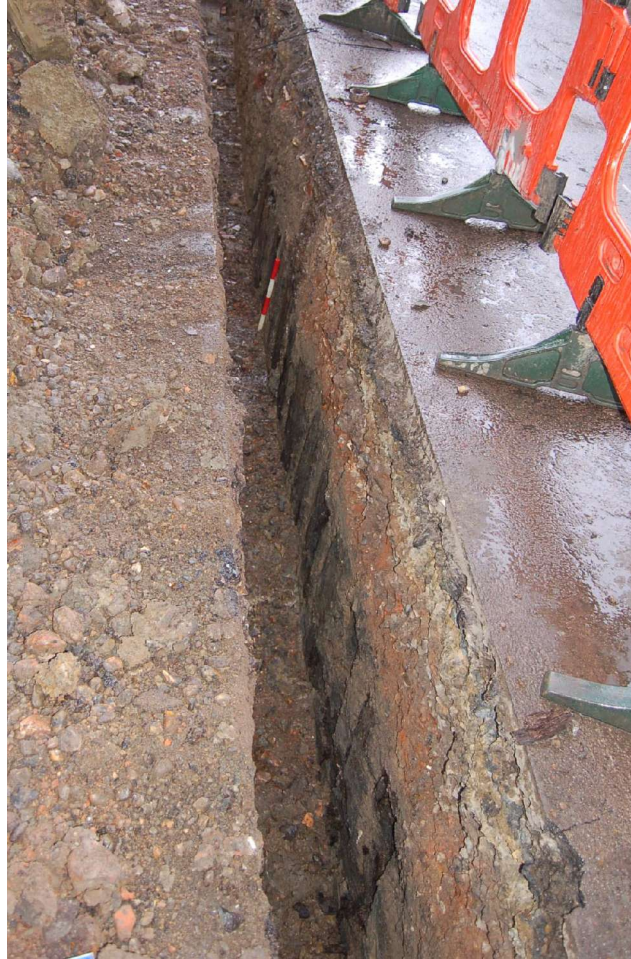
Figure 23: Looking East towards Priory Road, showing the line of upright timbers in section.
