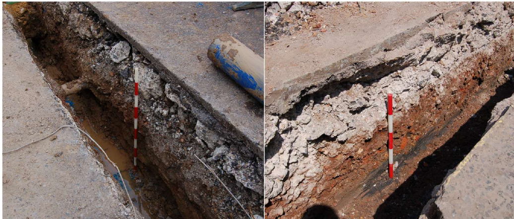
Figure 18: Sections of trenching on Priory Road (04-05-08 – northwest facing section, left and 09-06-08 – southeast facing section with chemical staining to the base of excavations, right).
