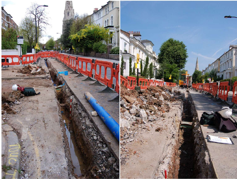
Figure 17: Trenching on Priory Road (04-05-08 – view north from the Abbots Place junction, top and 09-06-08- view north, bottom).
