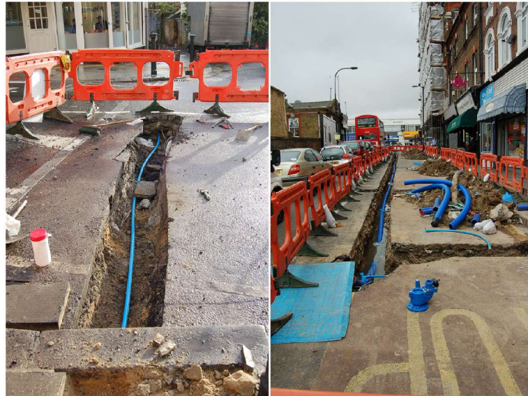
Figure 3: Trenching on Belsize Road (5/12/07-Trench A left and 28/05/08 – towards Kilburn High Road right).
