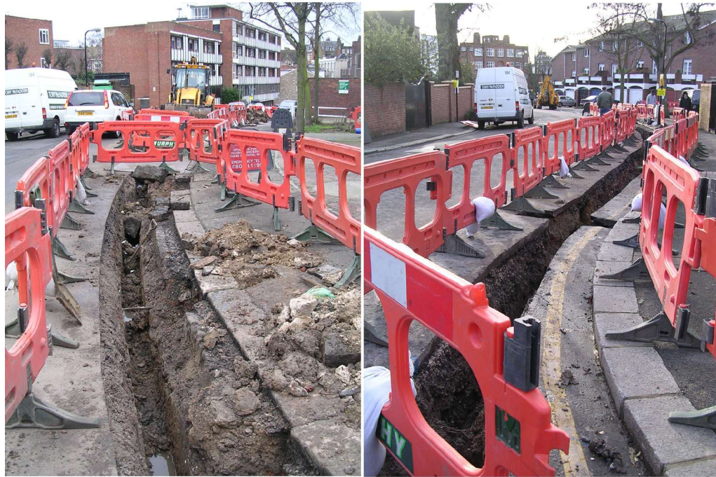
Figure 6: Trenching on West End Lane (17-01-08 – looking south, top and 09-01-08 – looking south, bottom).
