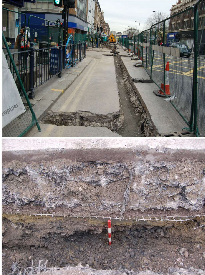
Figure 11: Trenching on Kilburn High Road (06-03-08 – view looking southeast, top and southwest facing section bottom).
