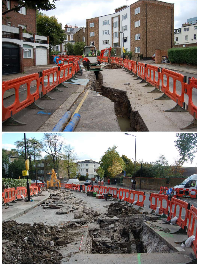
Figure 7: Trenching on West End Lane (20-08-08 – view north, top and 22-10-08 – West of Abbot’s Place, north end, bottom).
