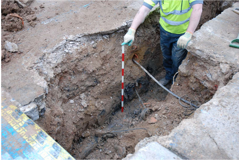
Figure 15: Example of trenching on Bransdale Close showing existing tarmac over concrete with service deposits and made-ground beneath.
