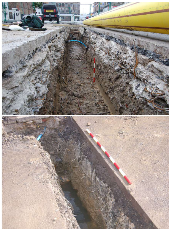
Figure 13: Trenching on Quex Road (18-03-08 – looking south, top and 01-04-08 – northwest facing section, bottom).
