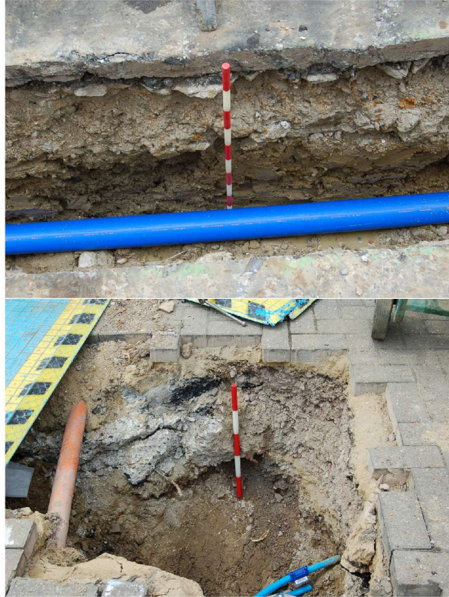
Figure 4: Exposed deposits in trenching on Belsize Road (28/05/08 – northwest facing section – top, and 25/07/07 – north facing section – bottom).
