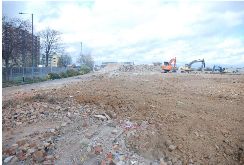
Figure 4: View looking north of Quadrant A after demolition and clearance, Great Cambridge Road runs parallel to the site in the left hand side of the photo.
