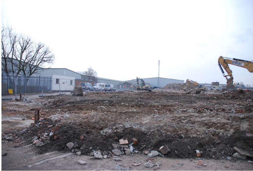
Figure 19: View southeast of Quadrant D showing the adjacent access road in the left of the photo.
