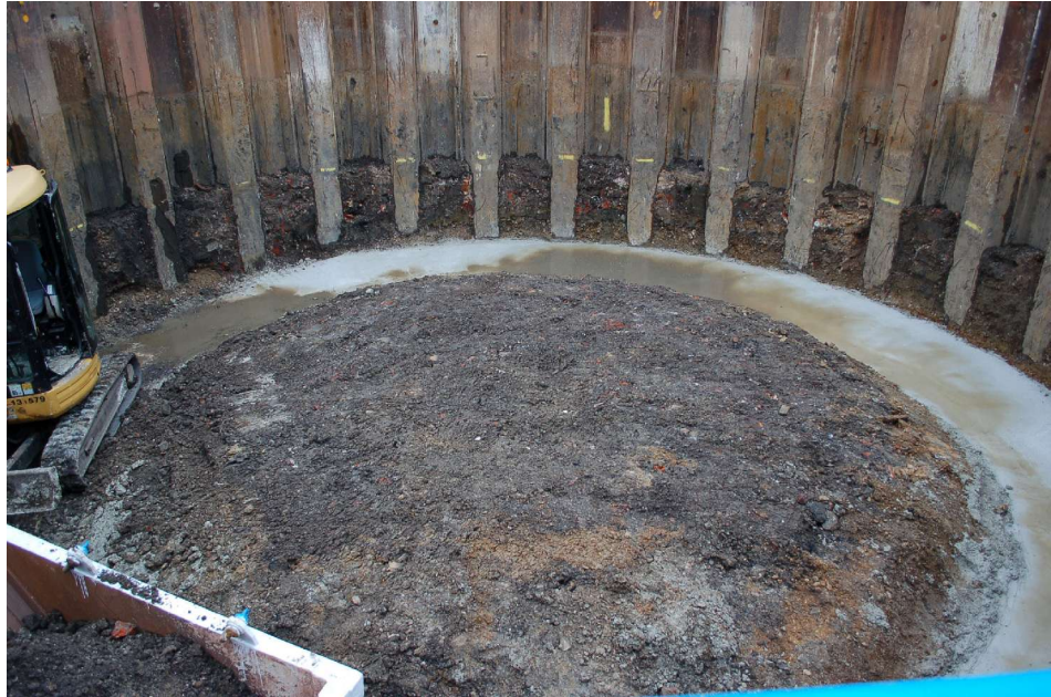
Figure 10: The central area designated for hand investigation following machining and laying of concrete in the outer ring.
