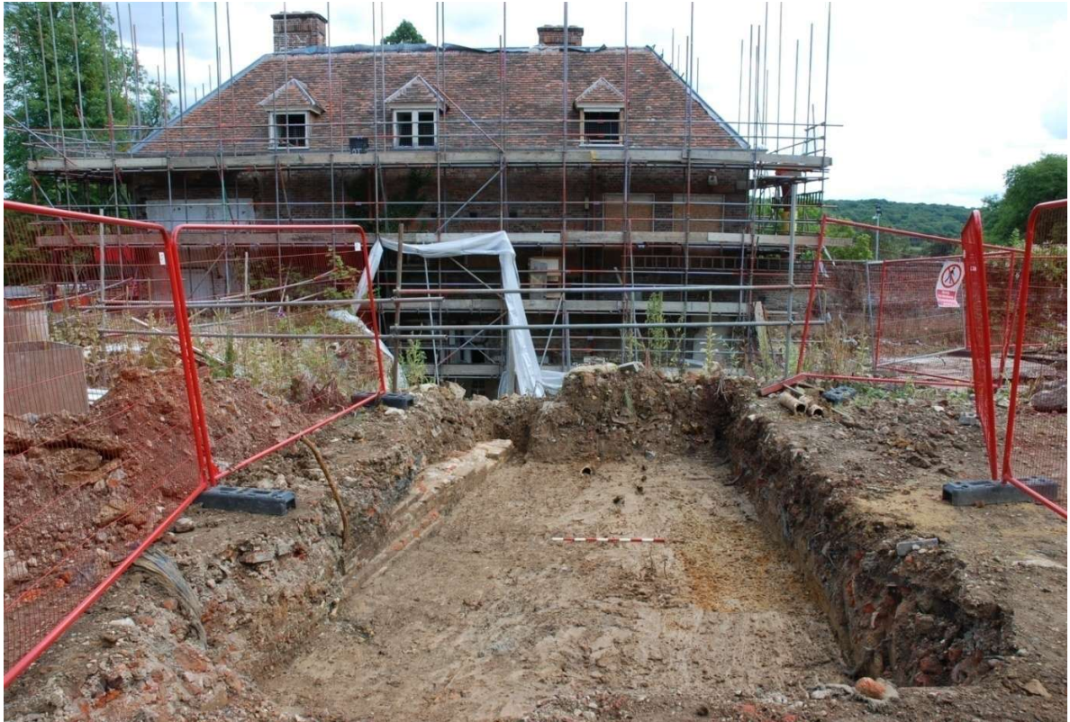
Fig. 36: Overview of Trench 6 looking southeast, with the brick wall base [2] to the left of the 1m scale
