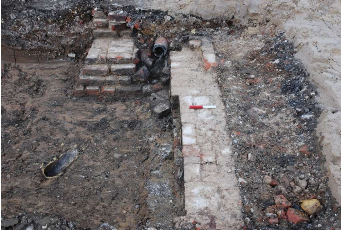
Fig. 26: Trench 4, view northwest along the brick wall base [10] that formed the front wall of the stable block, plus the remains of drain [9] ( scale 0.2 m ). The drainpipe cut into the brickwork near the top of the picture is a later and apparently unrelated feature
