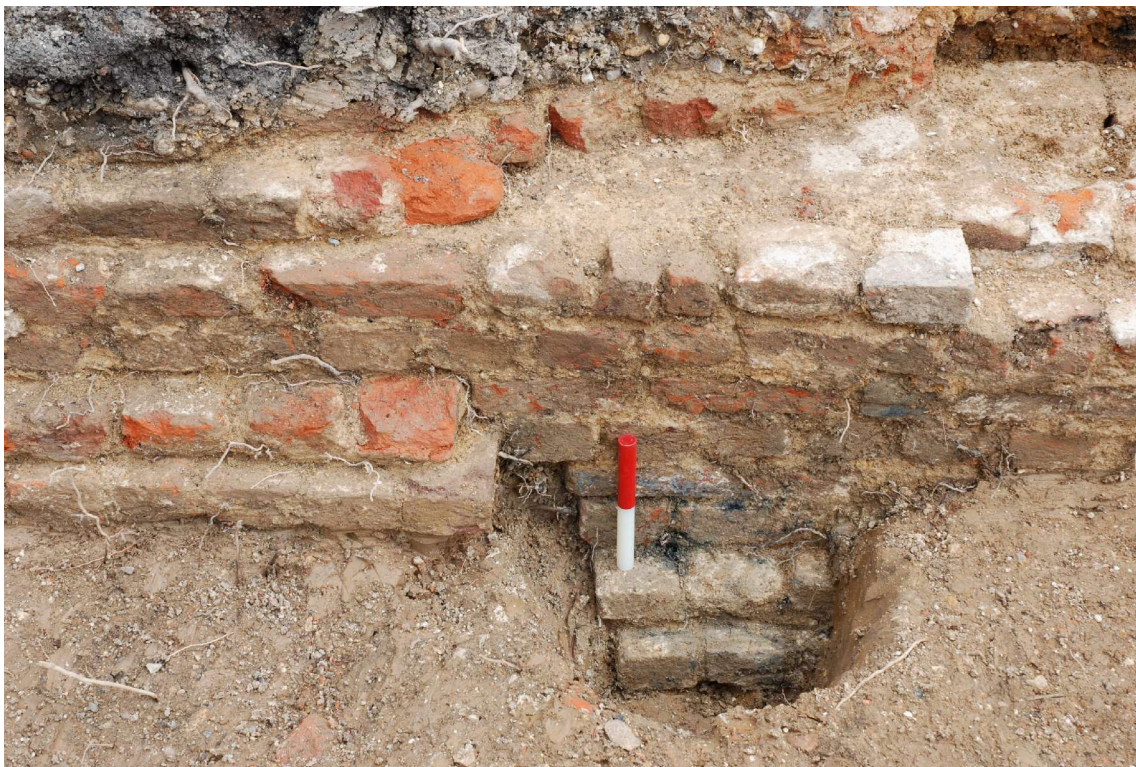
Fig. 39: Trench 6. Detail of exposed face and stepped base of the central section of wall [2] ( scale 0.2m ). The change in level and deeper footing to the east may simply reflect the proximity of the southeast corner of the building.
