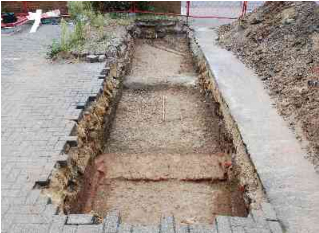
Fig 13 Trench 1: general view looking southeast towards Tooting High Street, with brick wall base [1] in the foreground ( 1.0m scale )
