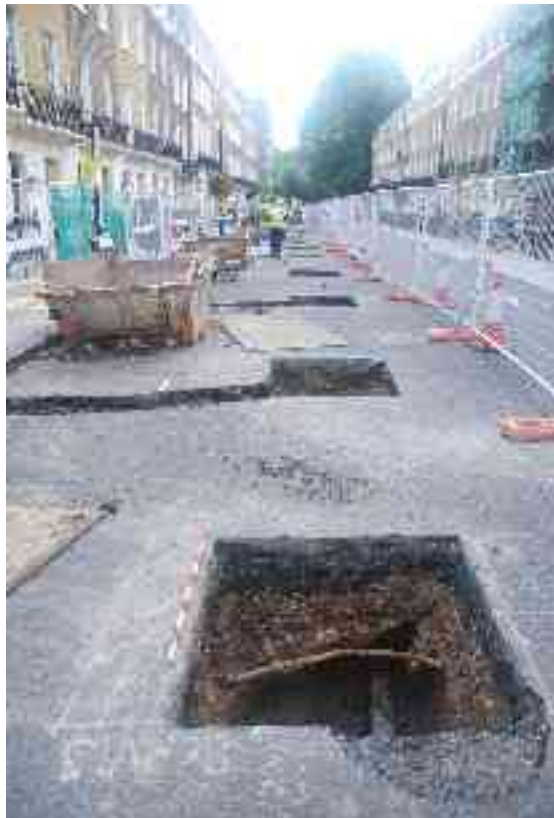
Fig 11 VMR works on Albion Street looking south towards Bayswater Road, showing the trenches and feeders (1m scale).
