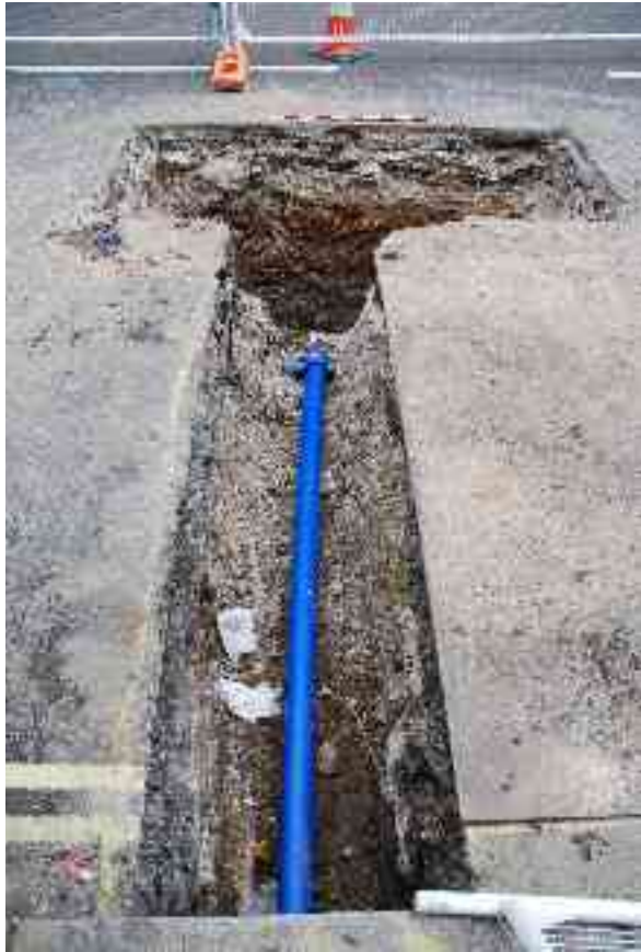
Fig 10 An example of the shallow feeder trenches that ran from the north kerb of Connaught Street, taken outside No 18 Connaught Square and looking south ( 1m scale ).
