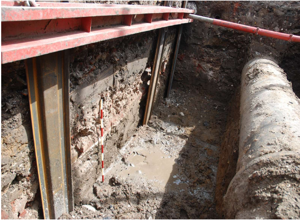
Fig 13 Detail of the lower half of the south facing section of Trench 2 prior to removal of the watermain.
