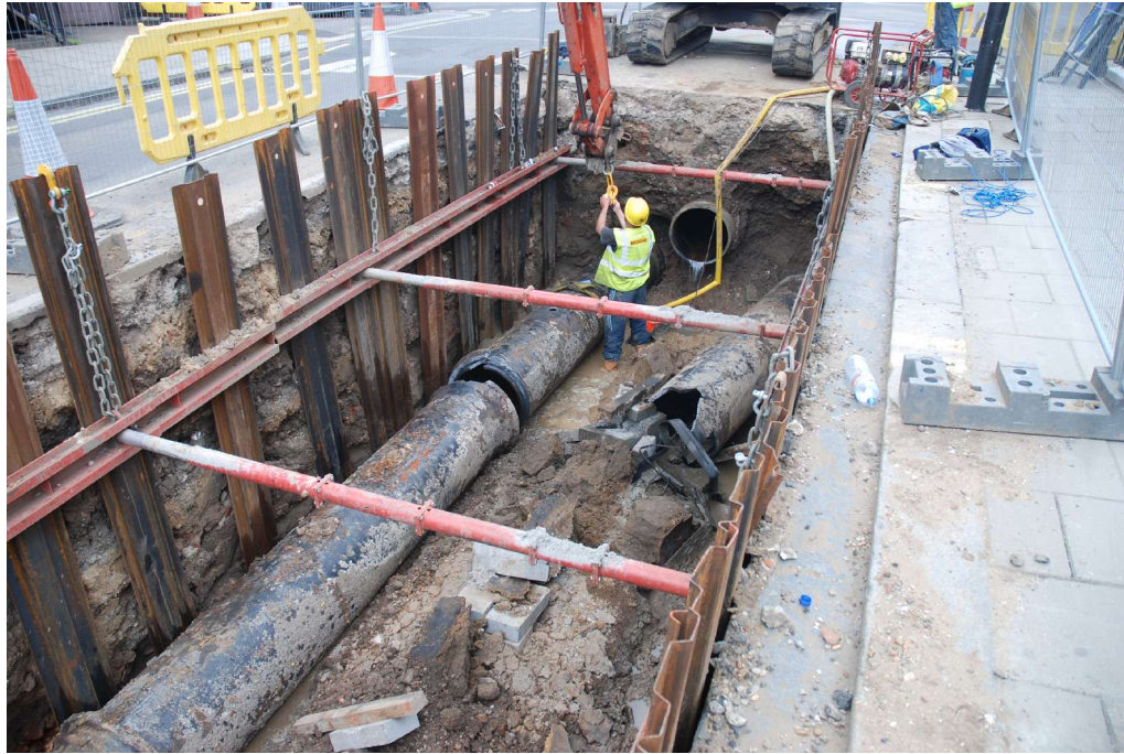
Fig 15 General view of Trench 2 after the pipe had been disconnected. The pipe was in places resting on top of a roughly constructed brick wall, which appears to have been constructed when the pipe was in place as the mortar was splaying out of the joints very noticeably on the northern side of the wall. The wall was evidently contemporary with the pipe in this area.
