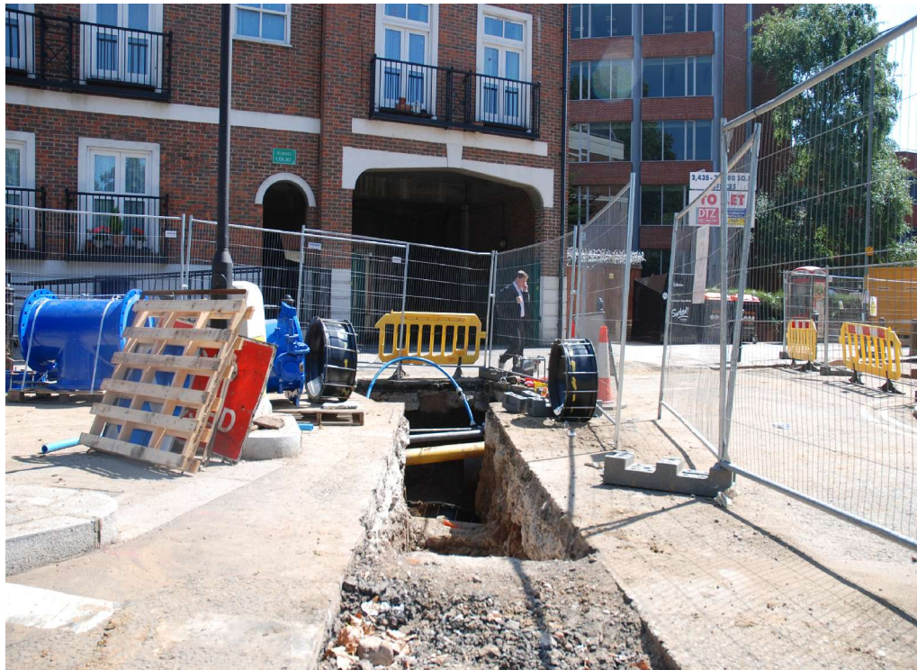
Fig 23 East of Putney Bridge Road and West of Simms Court, barriers for Trench 1 can just be seen to right of image
