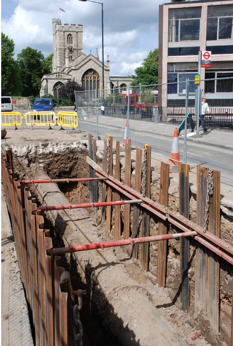
Fig 12 General view of Trench 2 on Gonville Street, looking west towards the parish Church of All Saints.
