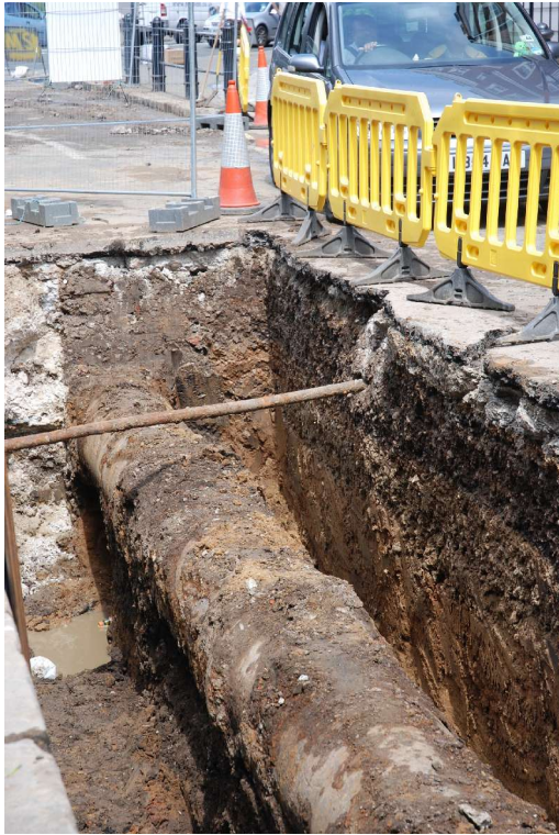
Fig 10 Detail of Trench 1 looking north and showing the west facing section of the trench on Fulham High Street. The stratigraphic layers can be seen: at the top the road make up layers of tarmac and concrete hardcore; overlying the modern made ground deposits with the yellow natural brickearth appearing at a depth of circa 940mm in the section at a height of +3.24m OD.
