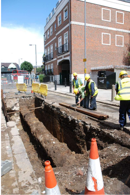
Fig 9 View of Trench 1 after excavation to the original watermain, looking north-north-east towards Simms Court.
