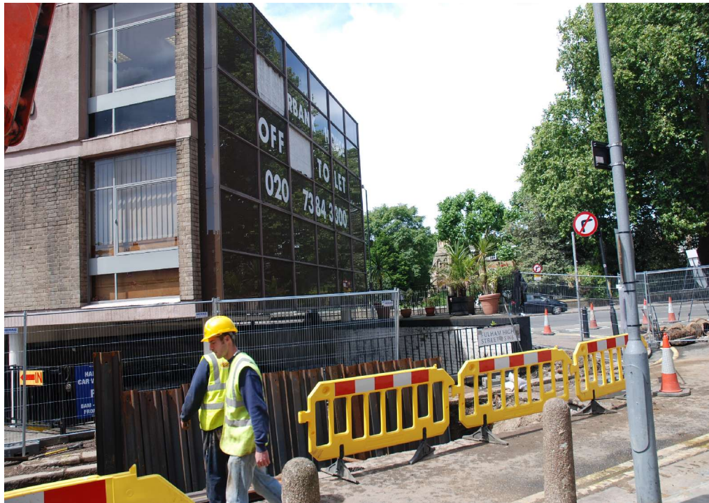
Fig 6 General view of Trench 1 on Fulham High Street, looking northwest towards the vicarage gardens across Putney Bridge Approach. The building to the left is Riverbank House (also known as Bridge House North), no. 1 Putney Bridge Approach. Trench 3 can be seen in the distance at the junction with Putney Bridge Approach (right).
