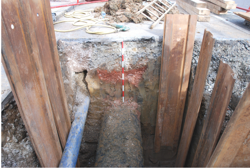
Figs 2 & 3 Views of the excavated pit looking east ( top ) and west. In both the 1m scale rests on top of the existing 24" trunk main.
